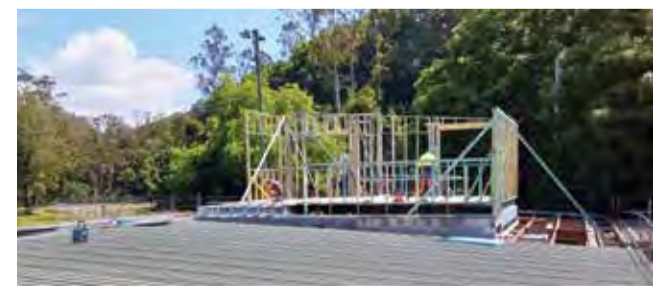
The upstairs meeting room is taking shape at Vic Bianchetti Sports Clubhouse at Uki.
