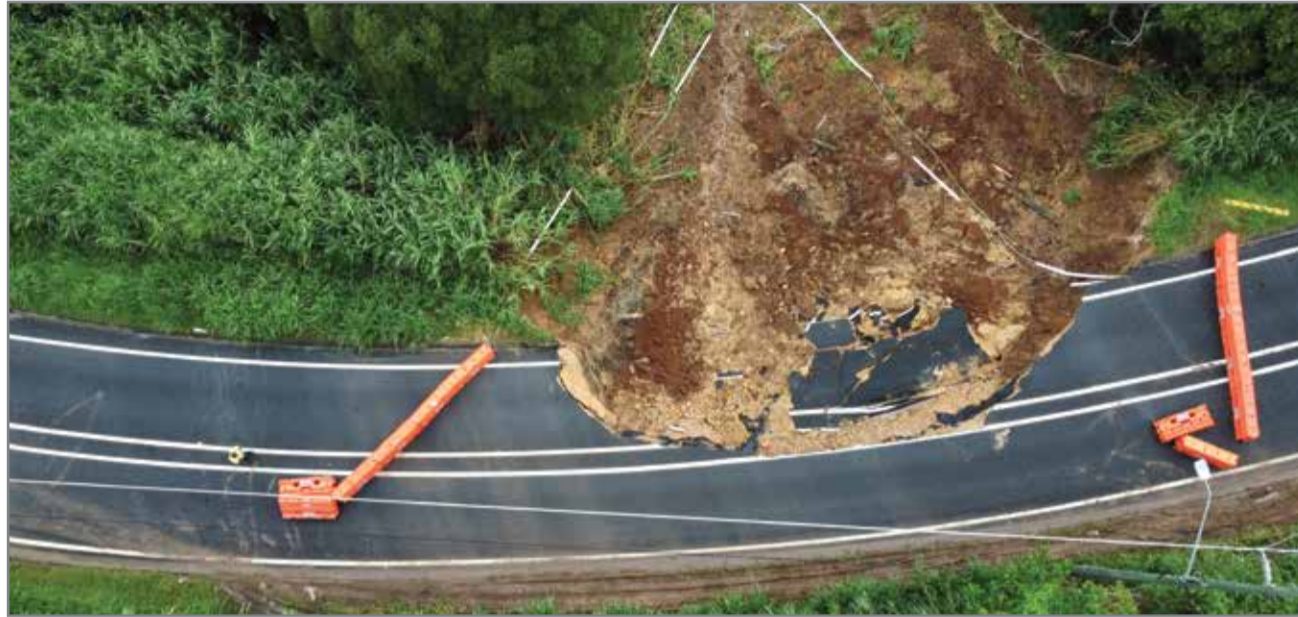
Scenic Drive at Bilambil Heights is closed due to a major landslide caused by the recent flood event.
