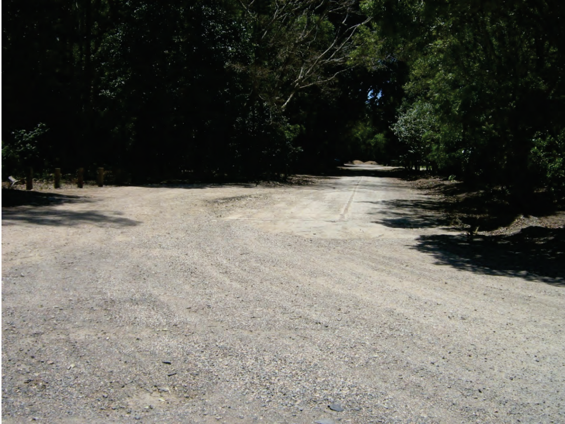
Figure 5: Potholed access road
