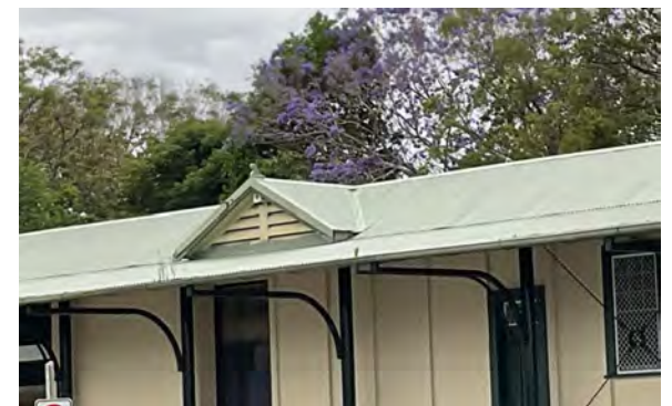
Picture 13 Missing fixing and lifting sheets, western elevation
