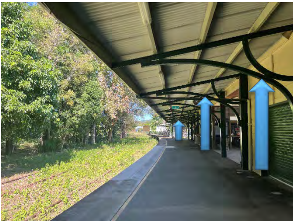
Picture 31 Indicative locations for three hanging signs to commercial tenancies on platform side of station
