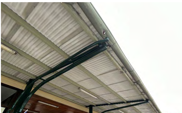
Picture 12 Dislodged downpipe and damaged gutter spikes, western elevation
