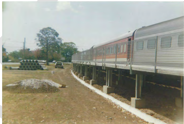
Picture 6 – Extended Platform and Carpark Works Source: NSW Railways Past and Present
