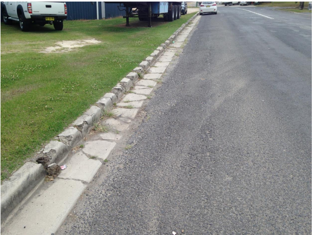
Figure 14 - Example Concrete Kerb Condition Score 5
