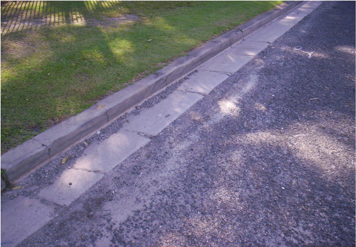
Figure 13 - Example Concrete Kerb Condition Score 3
