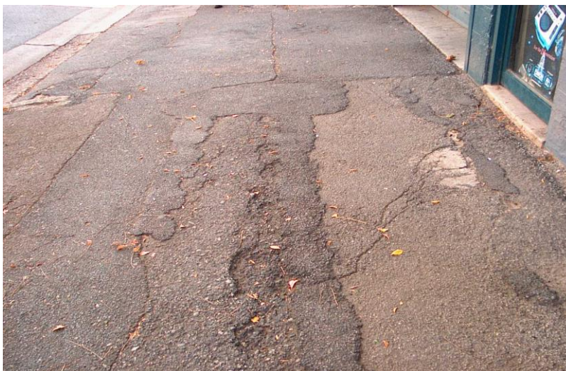
Figure 18 - Example Asphalt Footpath Condition Score 5
