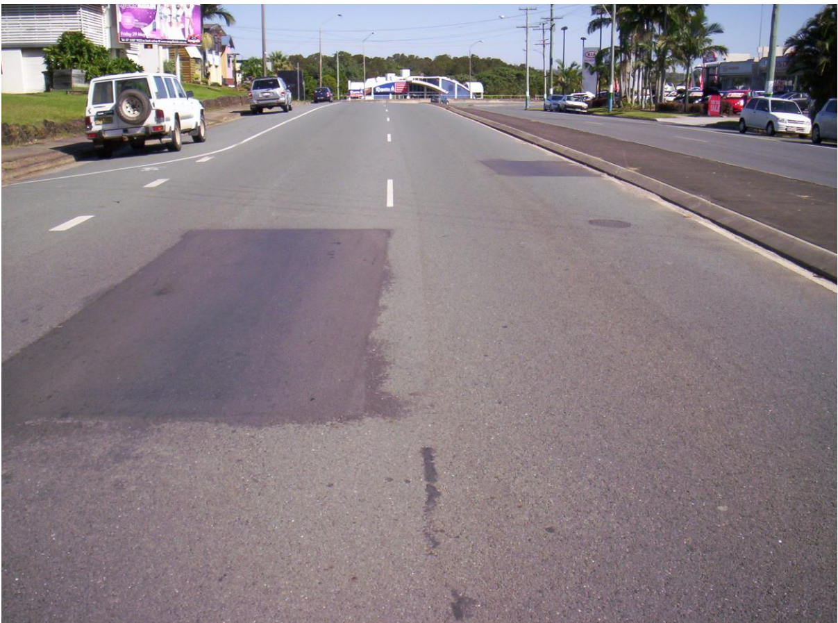
Figure 2 - Example Sealed Road Condition Score 3
