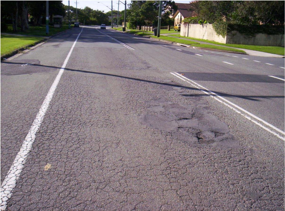
Figure 3 - Example Sealed Road Condition Score 5
