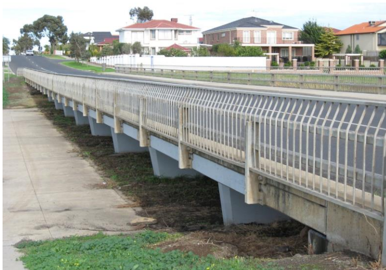
Figure 9 - Example Steel Bridge Rail Condition Score 3
