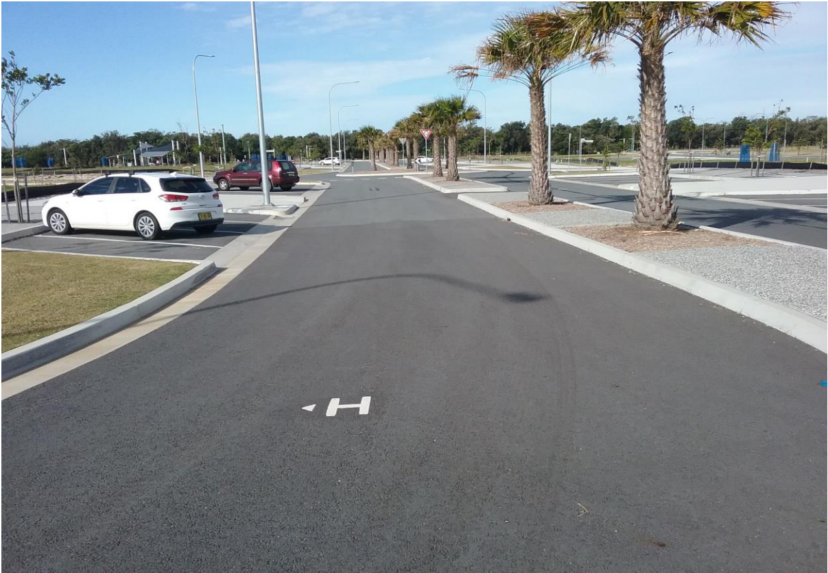
Figure 1 - Example Sealed Road Condition Score 0
