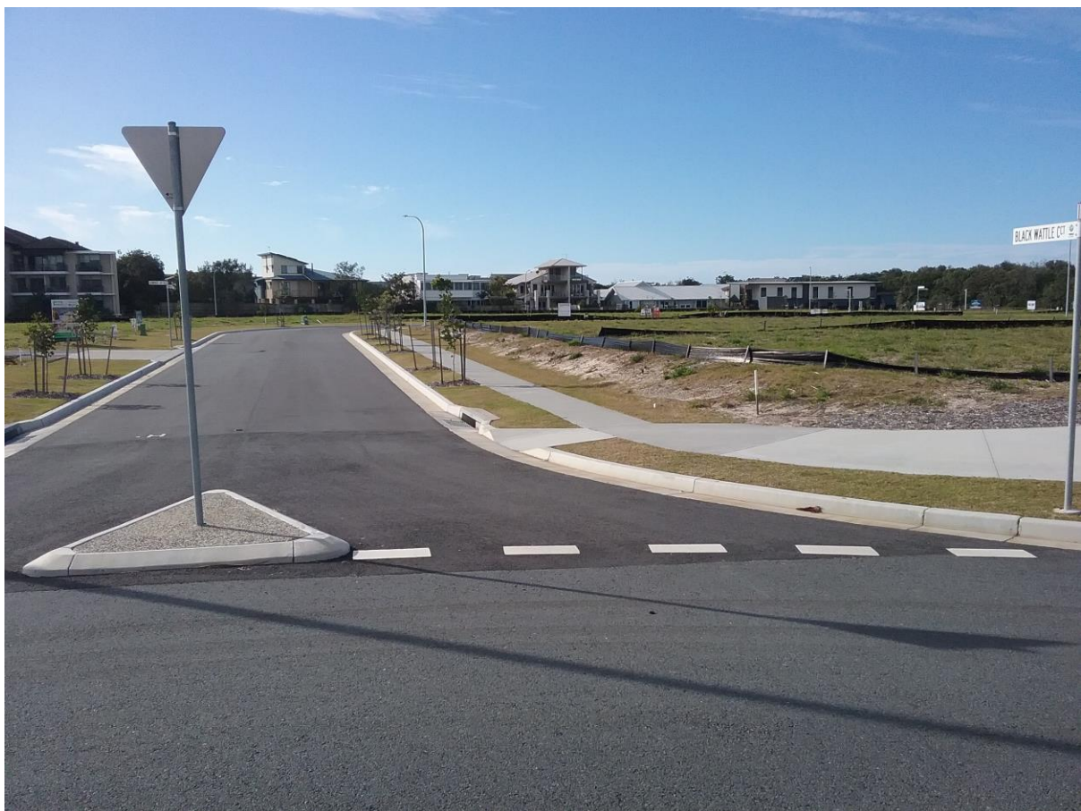
Figure 12 - Example Concrete Kerb Condition Score 0
