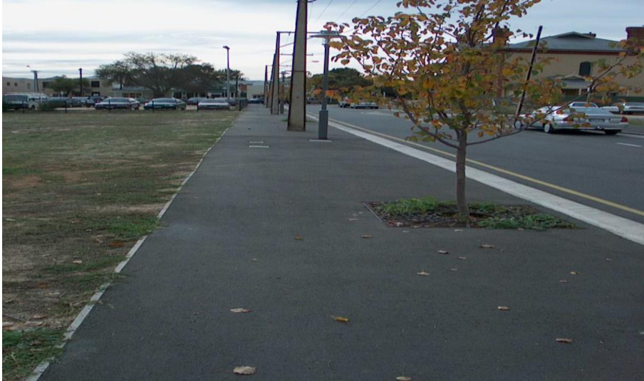
Figure 16 - Example Asphalt Footpath Condition Score 0
