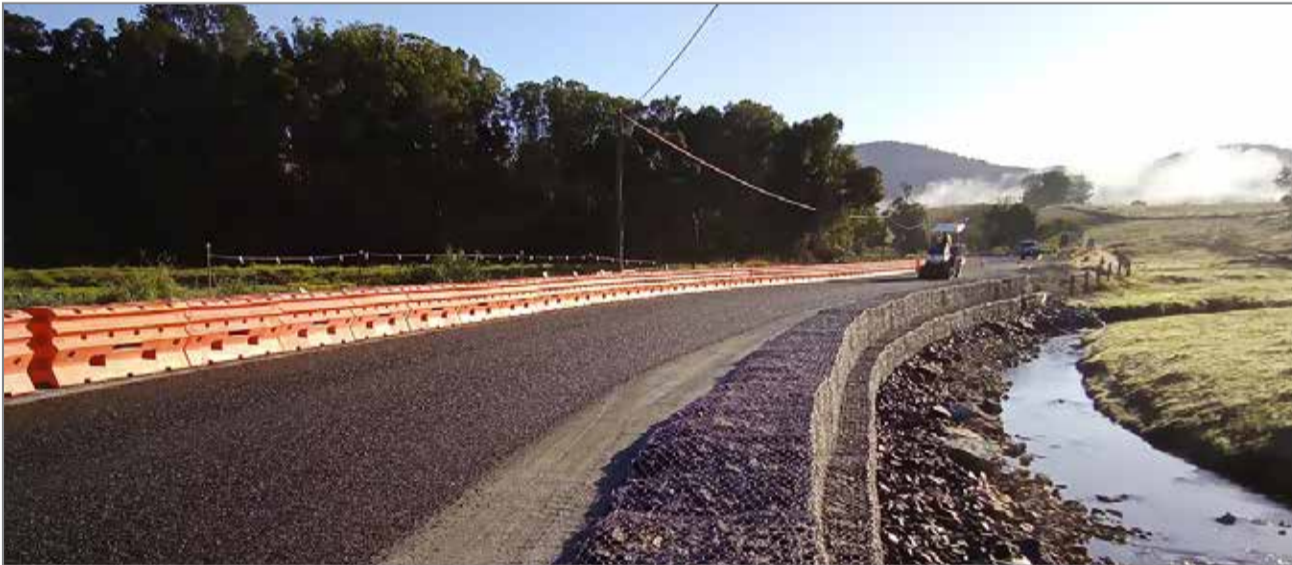
Tomewin Road was one of the many roads damaged in the flood 12 months ago and later repaired.
