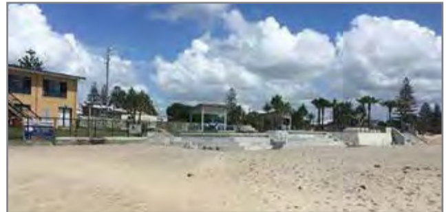
Minor works to repair the concrete seawall fronting Rowan Robinson Park at Kingscliff will commence next week.
