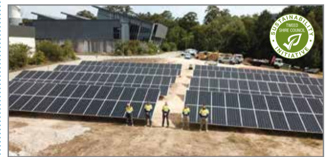
Council's first ground-mounted solar array at the Bray Park Water Treatment Plant helps power the treatment of drinking water.
