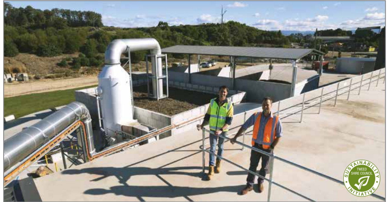
Soilco Operations Manager Michael Emery and Acting Project and Operations Officer Wes Knight at the new facility.
