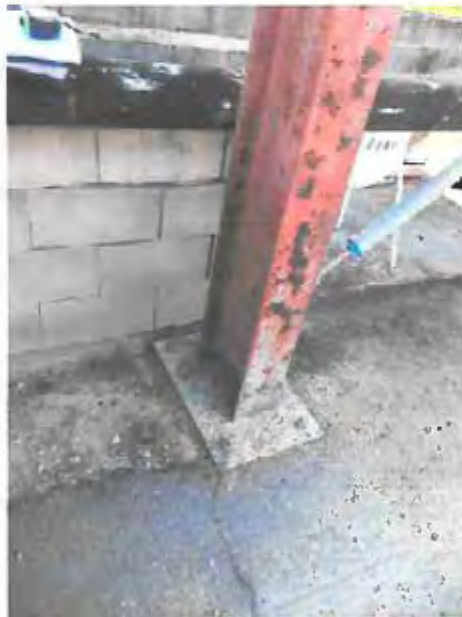
Figure 2 – Filling station column showing baseplate connection and surface rust
