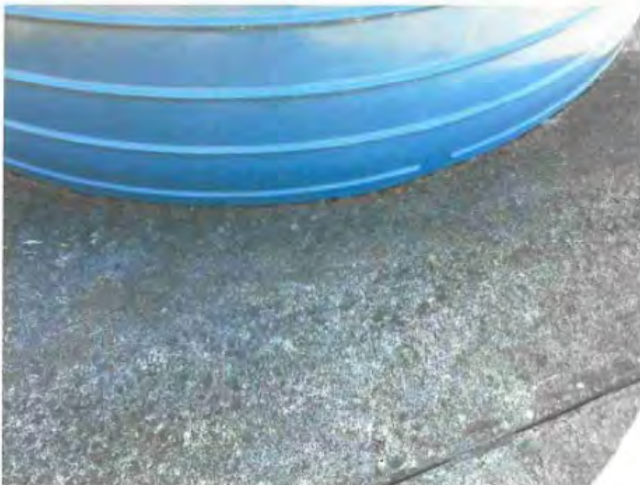
Figure 4 – Hairline shrinkage crack in tanks slab
