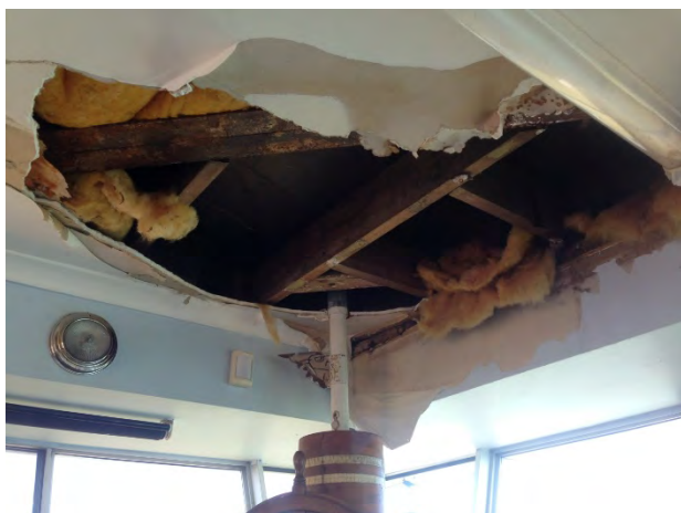
Photograph 2: Internal ceiling damage, first floor
