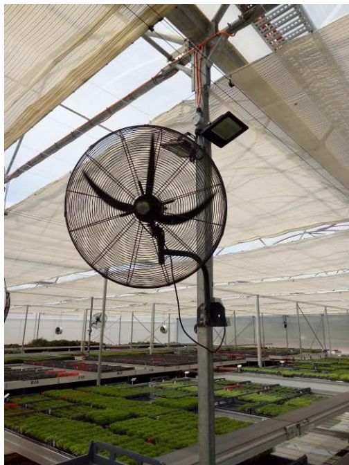
Photograph 3: Fixed Pedestal Fan
