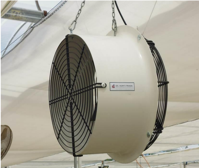
Photograph 1: HAF fans installed in the facility
