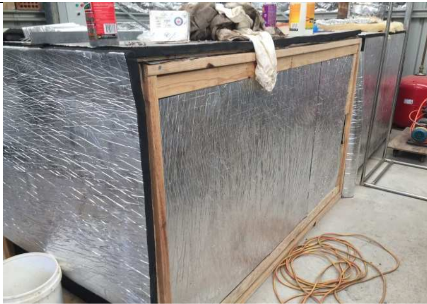
New Boiler Noise Insulated
