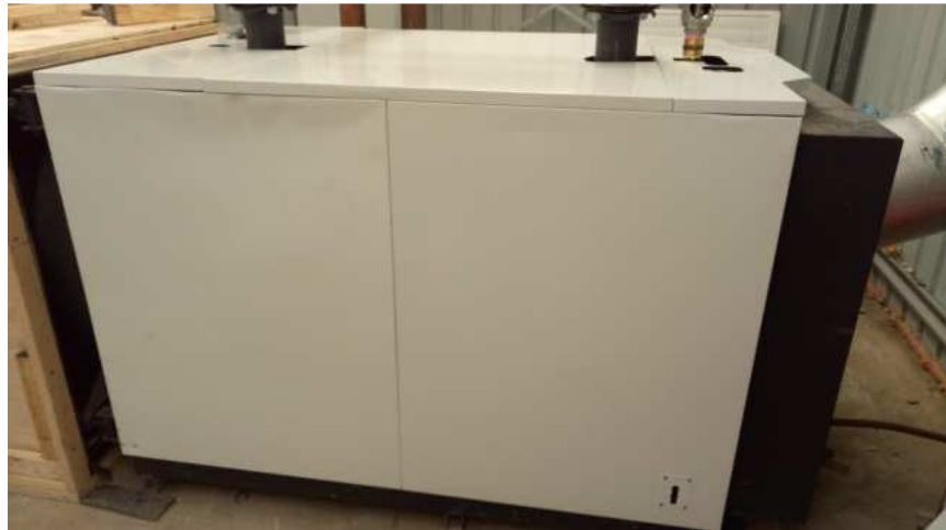
New Boiler Unlagged
