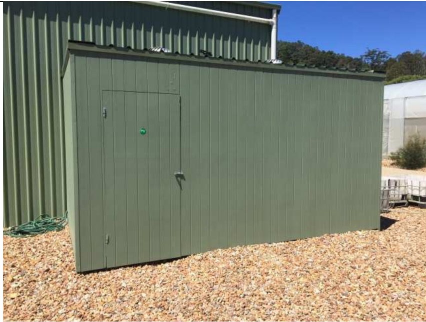
Generator Noise Insulated
