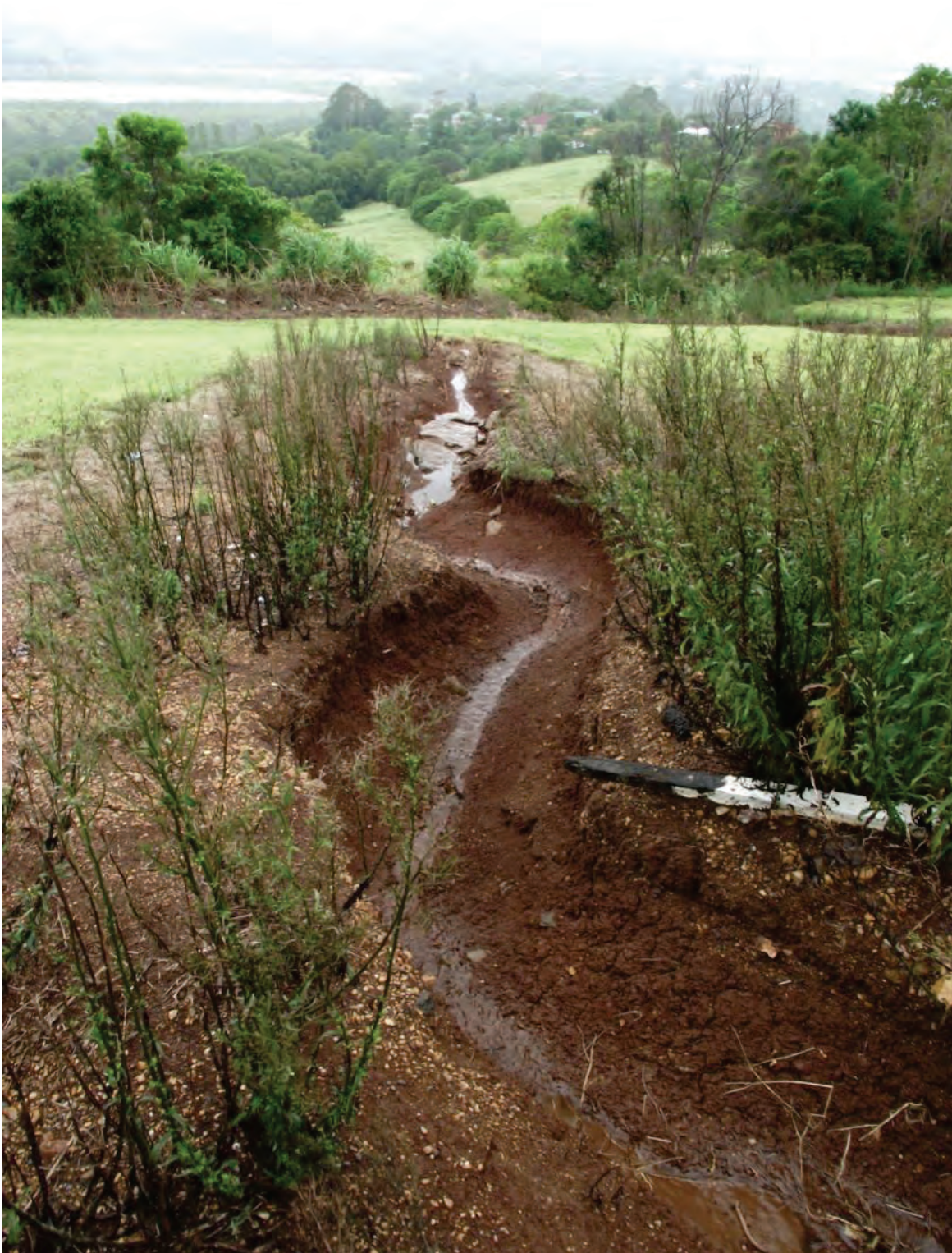
FIGURE 6: EXISTING SCOURED DRAINAGE LINE BELOW PIPE OUTLET UNDER TERRANORA ROAD
