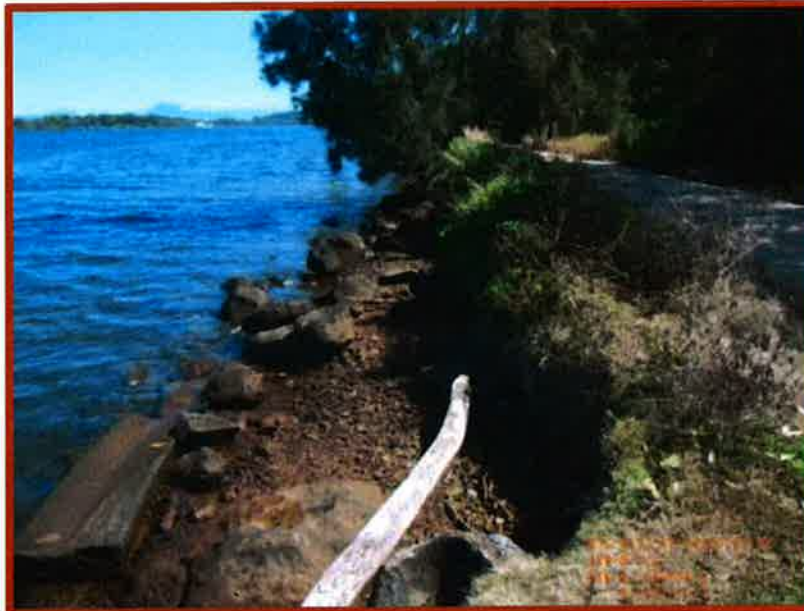
Figure B30 Severe erosion at upstream side of revetment at old Ferry Road
