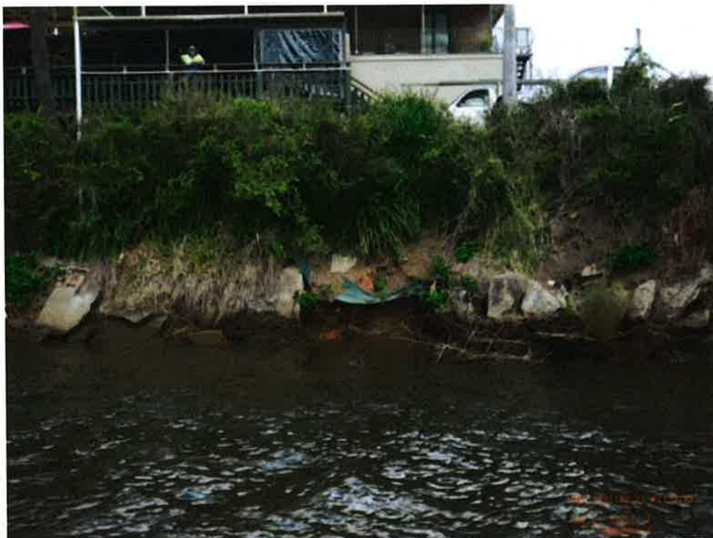
Figure A13 Photograph of an example section of river bank with ad-hoc river bank defences in place in the Tweed River.
