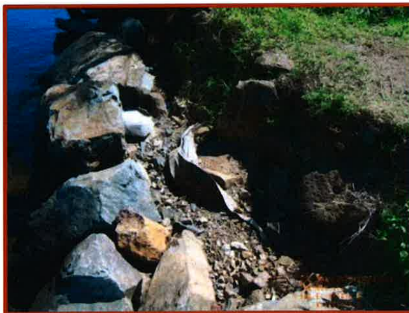
Figure B31 Severe erosion and failed revetment at eastern side of Oxley Cove adjacent to Bosun Boulevard
