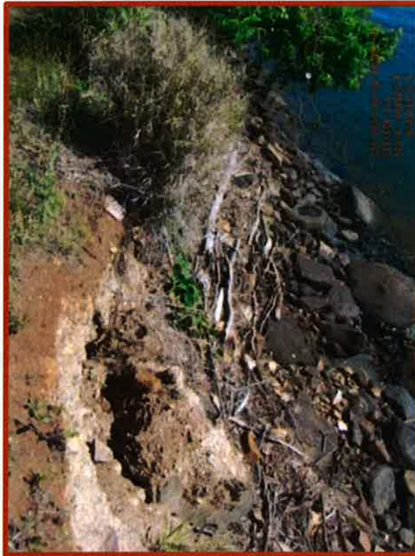
Figure B37 Section of embankment at Chinderah suffering erosion
