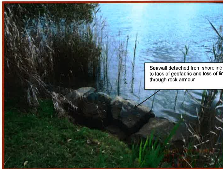
Figure B7 Detached section of revetment due to continuing erosion caused by lack of geofabric
