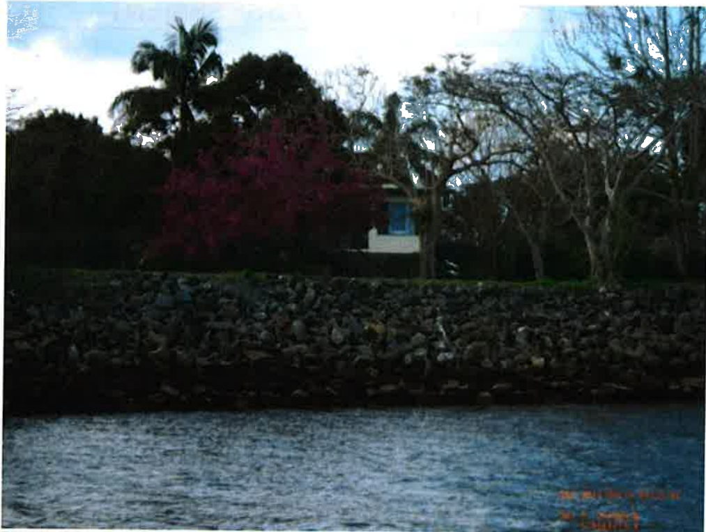
Figure A14 Photograph of an example section of river bank with a well designed rock revetment in place along the Tweed River.
