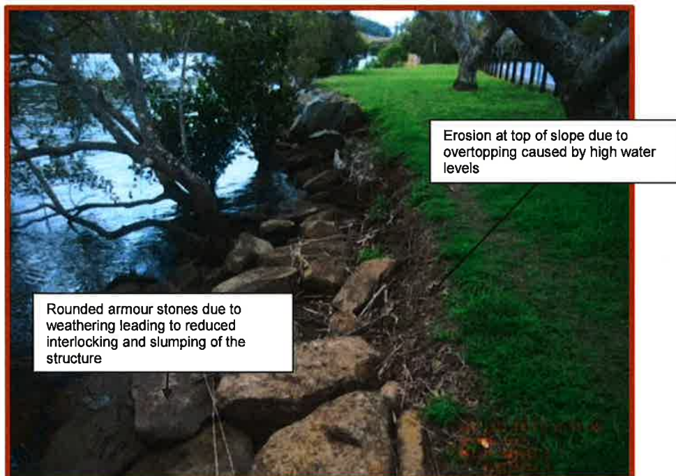
Figure B6 Erosion occurring at top of slope due to overtopping at a low-crested section
