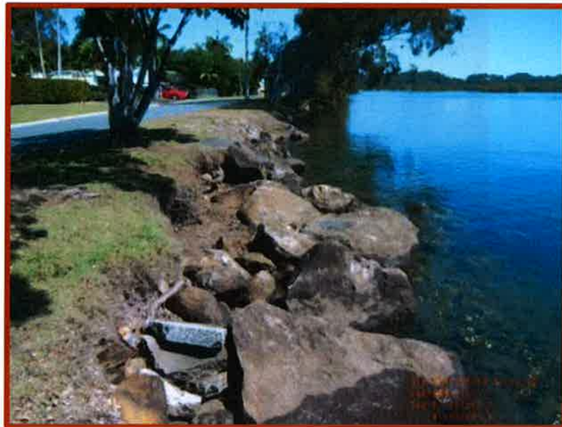
Figure B25 Severe erosion due to revetment overtopping and lack of geofabric underlay
