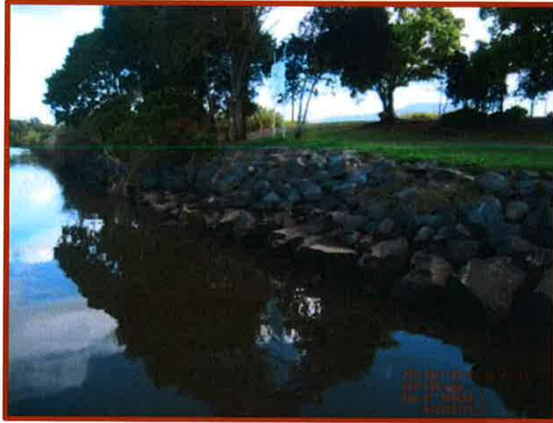
Figure B17 Revetment adjacent to boat ramp at upstream end of Commercial Road
