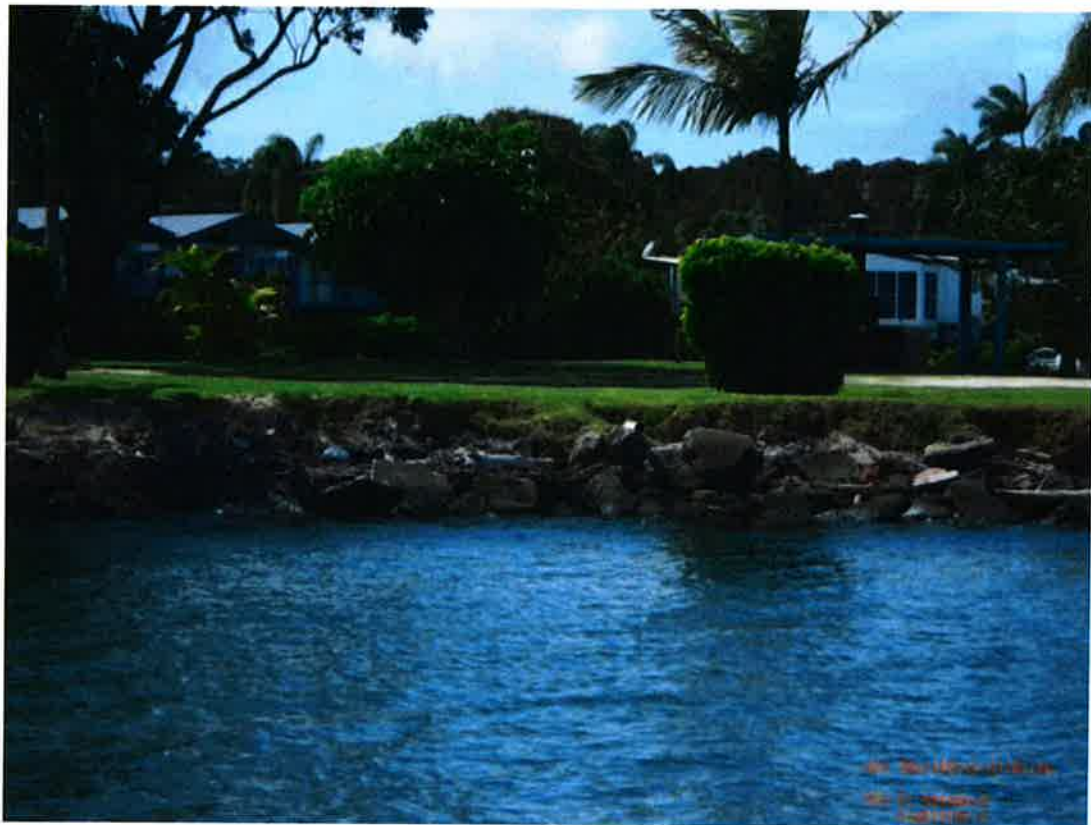
Figure A7 Photograph of a section within Map 5 which was previously recorded as eroding and now has ad-hoc poor defences in place.
