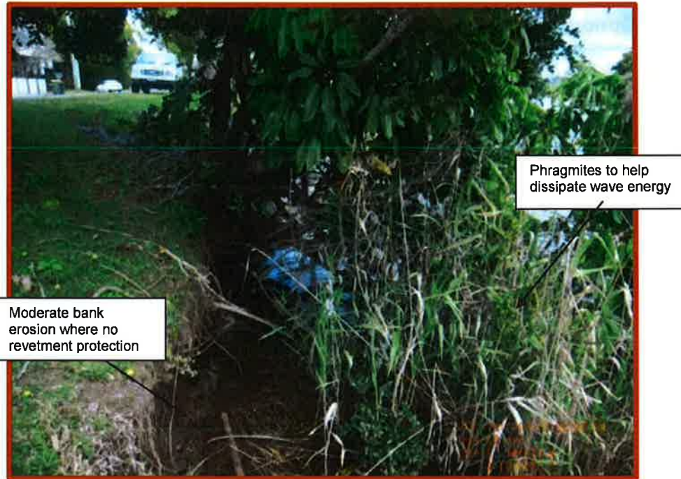
Figure B5 Eroded unprotected section at Tumbulgum foreshore
