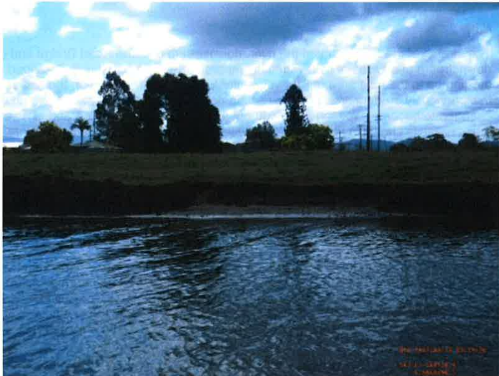
Figure A1 Photograph of the new area of erosion in Map 1.
