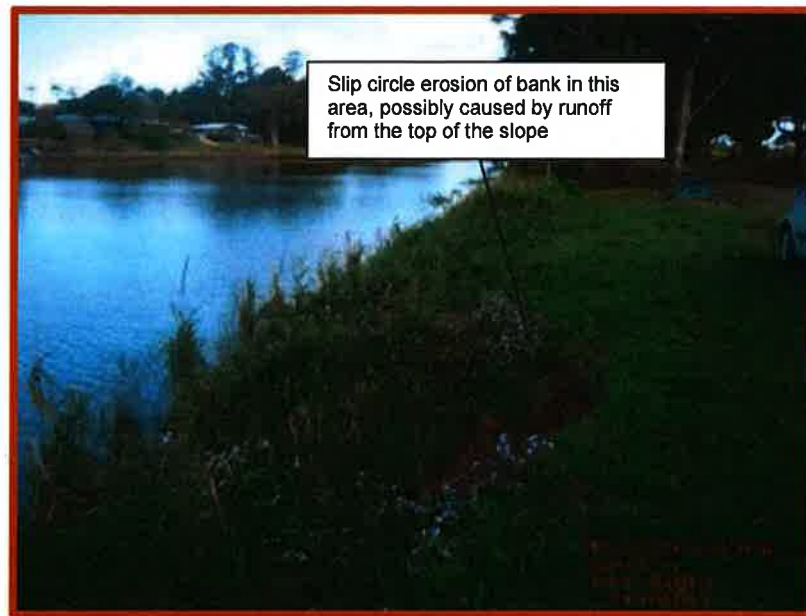
Figure B16 Erosion occurring upstream of Commercial Road area
