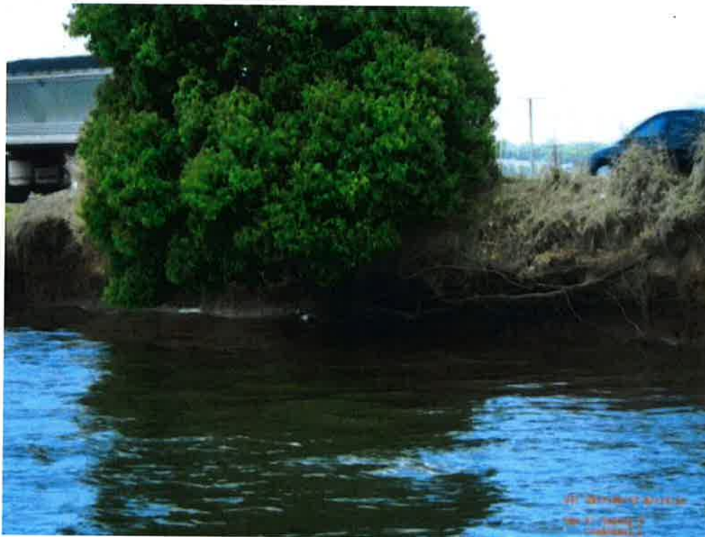
Figure A10 Photograph of an example section of river bank experiencing undercutting within the Tweed River.
