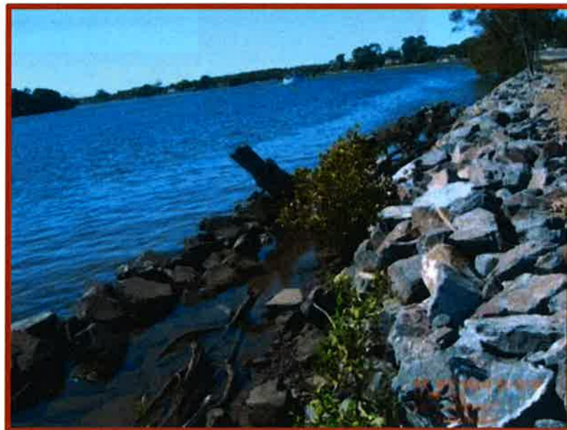
Figure B34 "Double wall" at Banora Point to encourage growth of mangroves along bank
