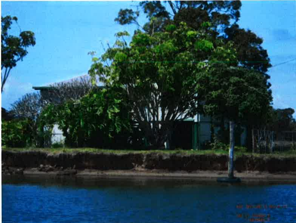
Figure A8 Photograph of an example eroding section of river bank within the Tweed River.
