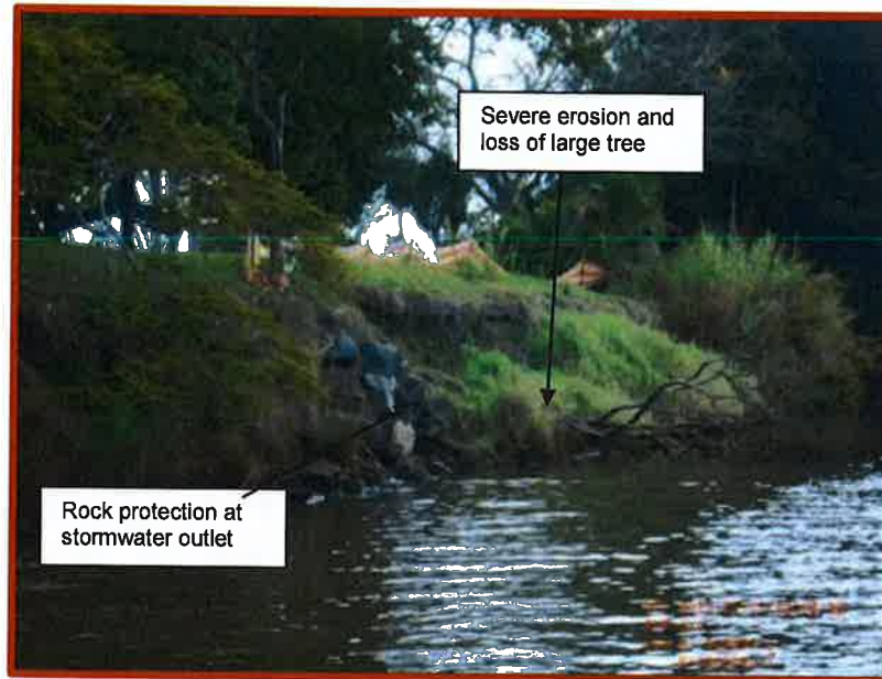
Figure B12 Severe erosion at Budd Park
