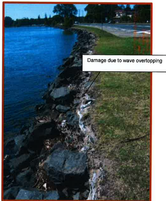
Figure B36 Revetment with insufficient crest width showing some damage due to overtopping
