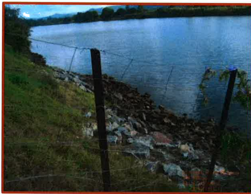
Figure B15 Revetment at South Murwillumbah Levee with slumping of toe rock and deformation of profile
