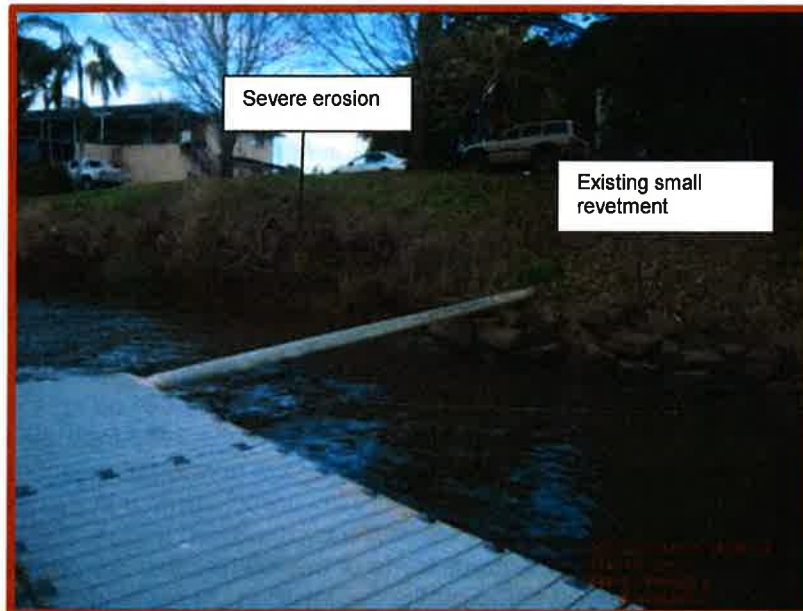
Figure B13 Existing revetment and adjacent erosion at Budd Park
