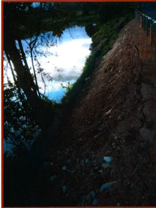
Figure B21 Unprotected embankment – Rous River (centre)
