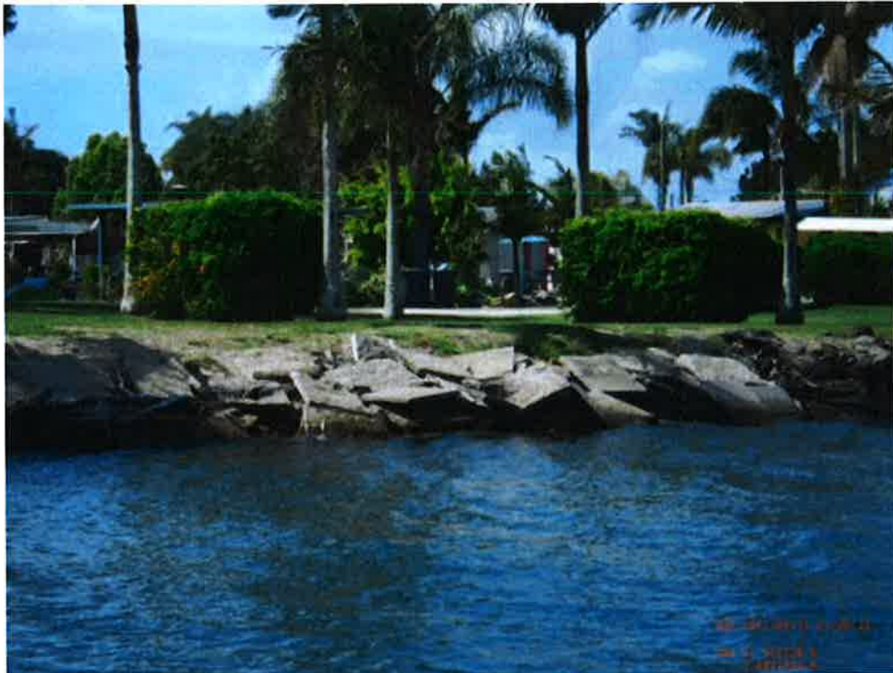
Figure A12 Photograph of an example section of river bank with ad-hoc river bank defences in place in the Tweed River.
