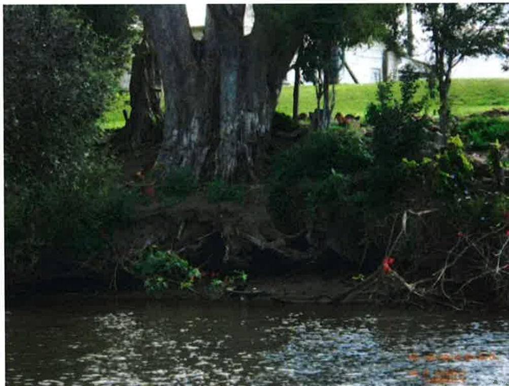
Figure A9 Photograph of an example section of river bank experiencing undercutting within the Tweed River.
