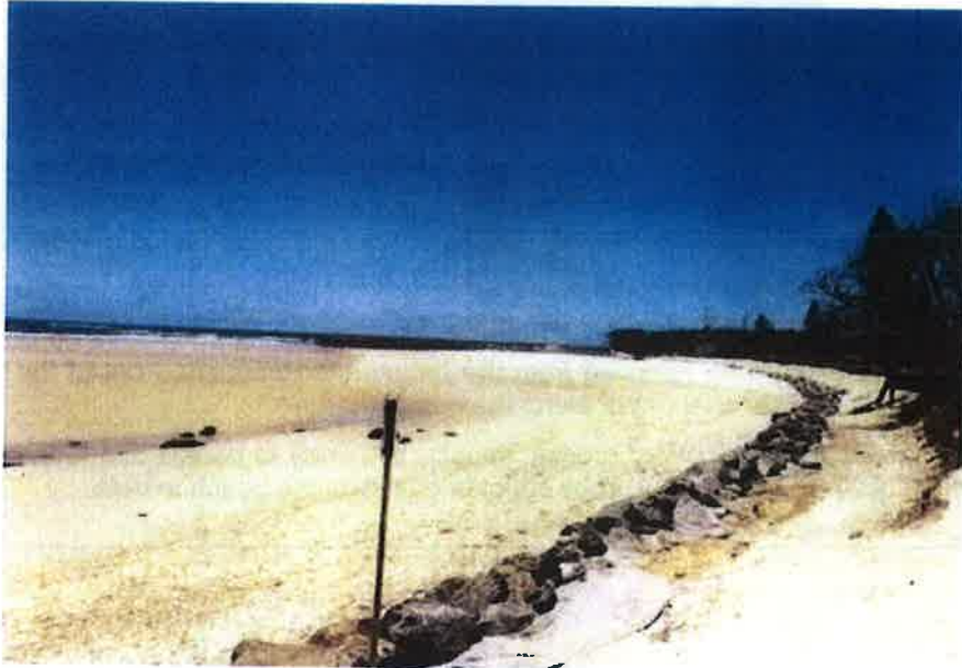
Figure 6 - Terminal rock revetment between Cudgen Headland SLSC and the Cudgen Creek training wall (present in the background). The photo shows the current sand pulse that has recently moved into the embayment and now resides at the southern end of the compartment in front of the wall. Photo M. Daley 8 November 2011.
