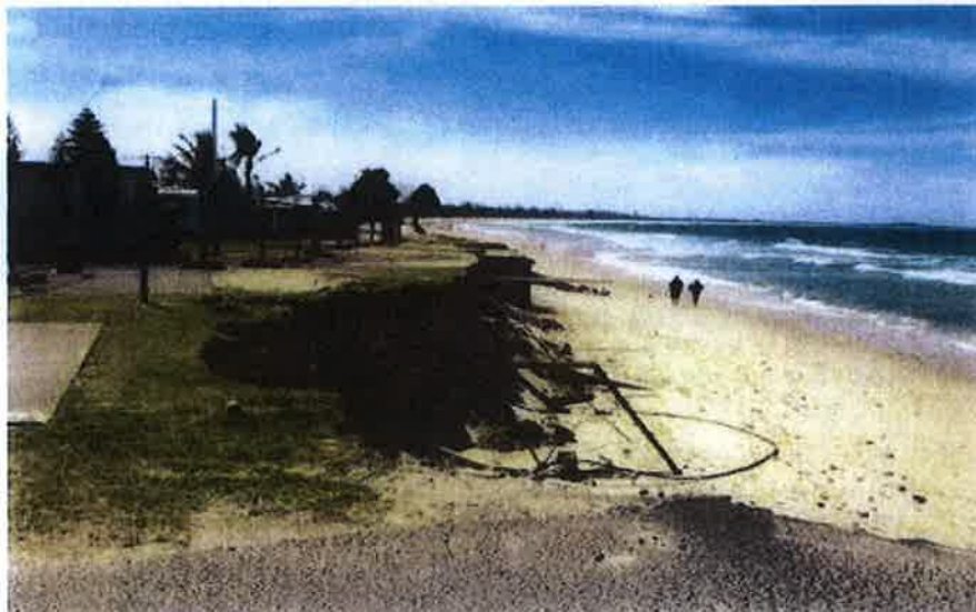
Figure 13 – Cable and Piping Infrastructure currently protruding from the erosion escarpment adjacent to the Holiday Park. Photo: M. Daley 8 November 2011.
