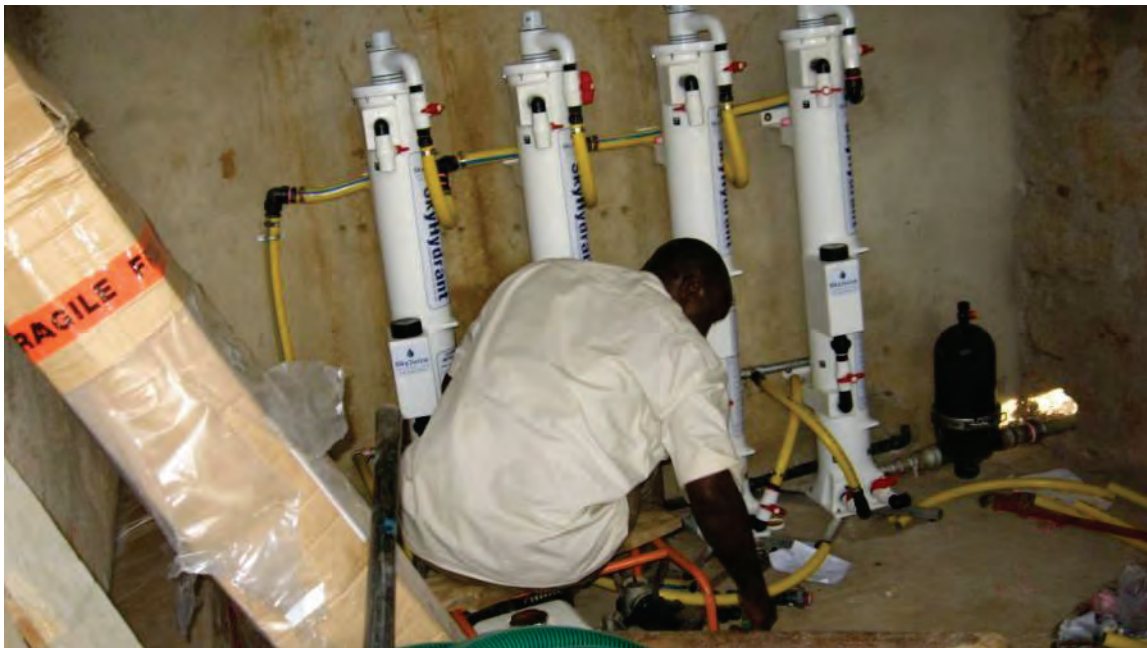
Figure 2. David Opondo, TKMP Program Manager installing SkyJuice water filters
