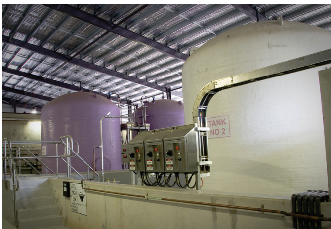
Storage Tanks within Facility
