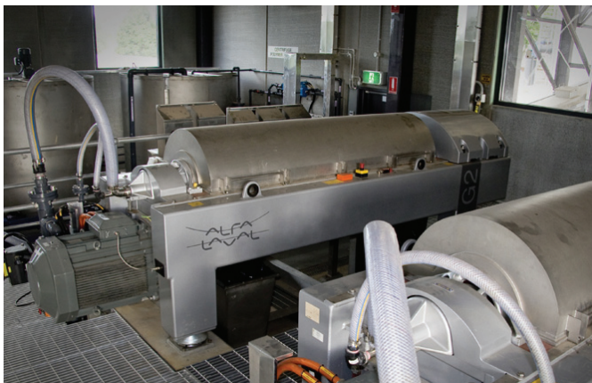
Centrifuges dewater the solids
