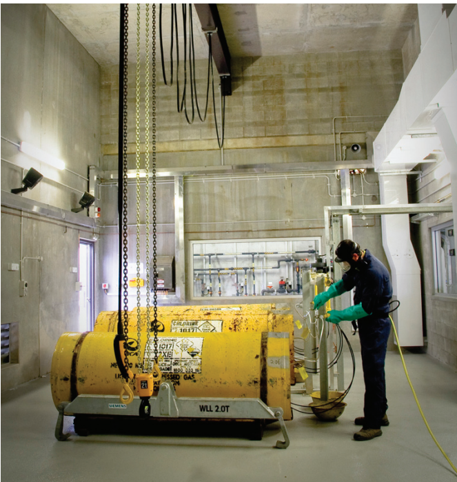
Chlorine Dosing Room
