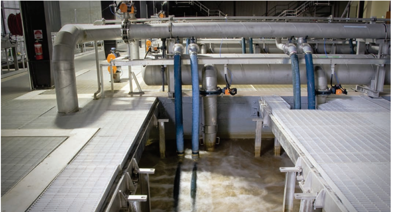
One of the four Membrane Tanks
