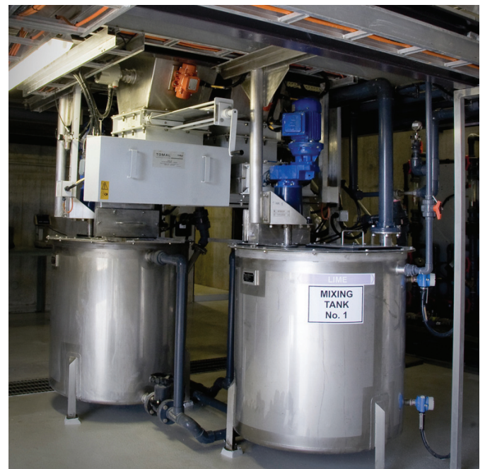
Lime dosing facility
