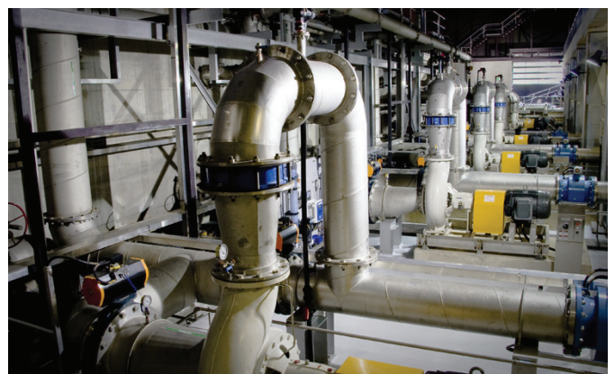
Permeate pumps within the pump gallery
