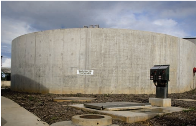
Sludge Thickener Tank
