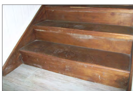
Stairs constructed using H3 treated timber and marine ply with lowest riser cover removable to allow underside of stair to be flushed easily. The wide internal stairs allow the easy move of belongings upstairs as the flood advances.
