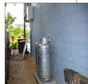
Electrical meter elevated above flood level (access platform under not yet fitted). Gas cylinders on slab poured with main slab and chained down. Core-filled besser block ground wall for flood flow resistance and easy clean.
