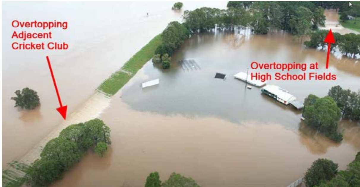
Plate 3 Overtopping of the Commercial Road Levee in 2022 Flood (image provided via YouTube by Offtopic: https://www.youtube.com/watch?v=UsPF5DTI44U )
