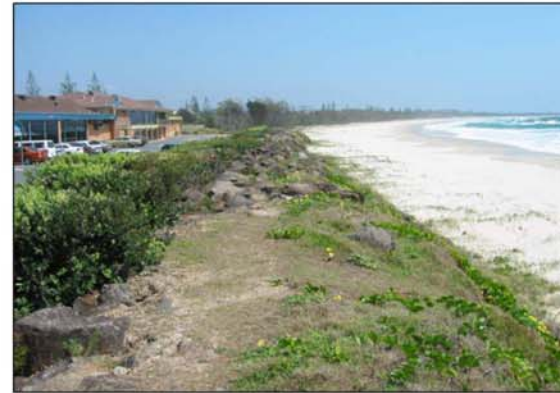
Existing BOWLS Club seawall looking north. The seawall is sparsely vegetated and partly buried with sand.
