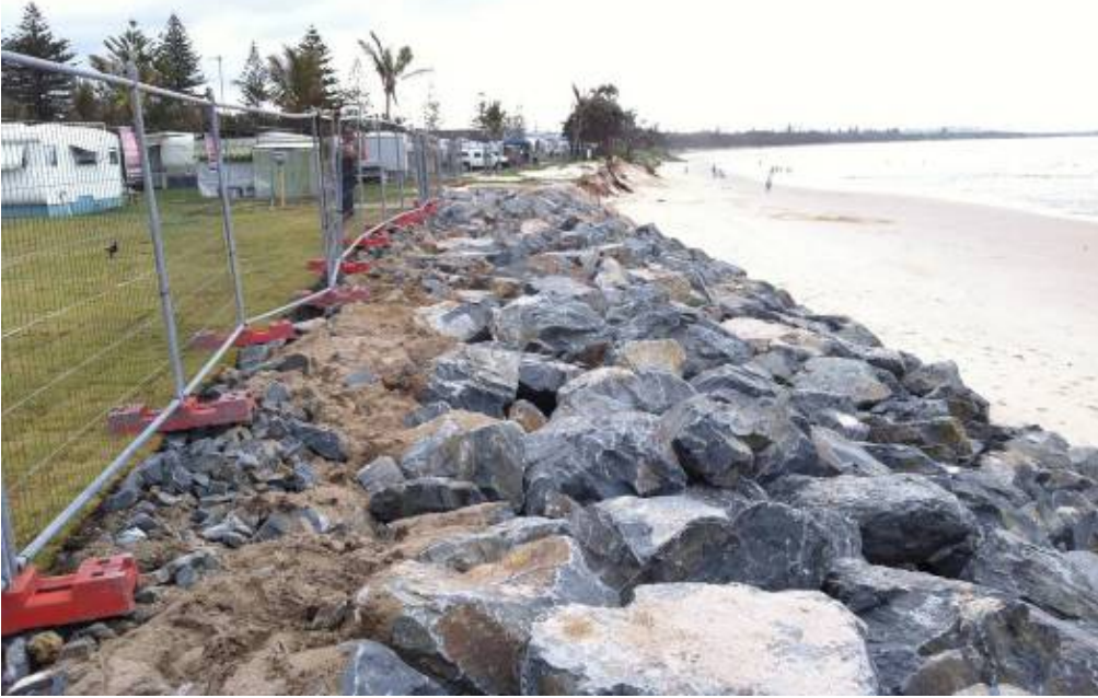
Figure 15 – Recent (December 2011) rock revetment works installed to protect the amenities block and sewer pumping station of the Kingscliff Holiday Park. Photo: B. Fitzgibbon 14 December 2011.
