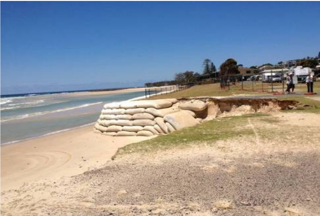
Figure 10 - Northern end of the geotextile sandbag seawall (looking south) showing both collapse of the wall and end effects which have produced further erosion of the Holiday Park. Photo: M Daley 8 November 2011.
