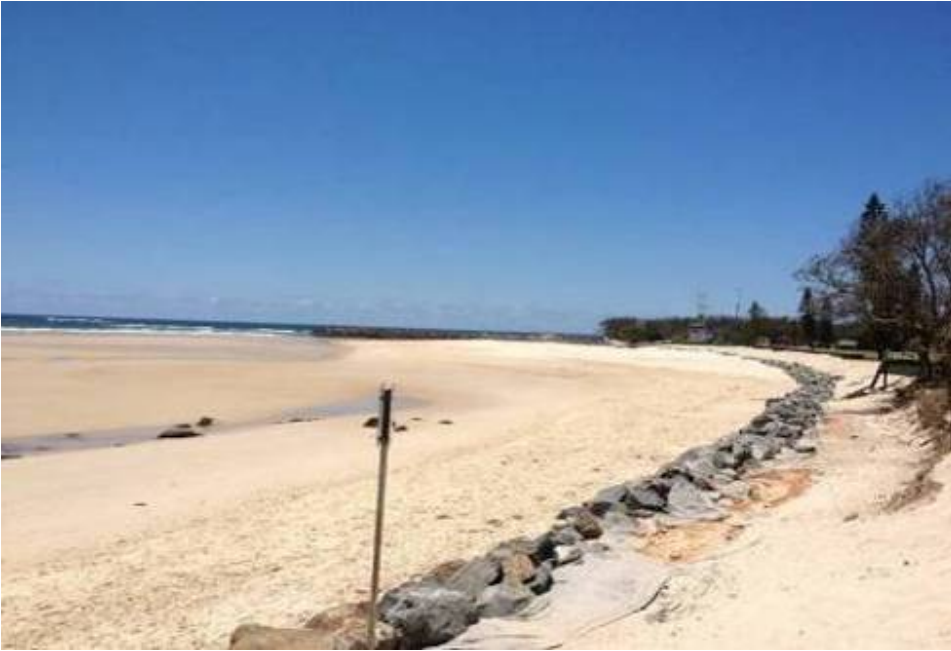
Figure 6 - Terminal rock revetment between Cudgen Headland SLSC and the Cudgen Creek training wall (present in the background). The photo shows the current sand pulse that has recently moved into the embayment and now resides at the southern end of the compartment in front of the wall. Photo M. Daley 8 November 2011.
