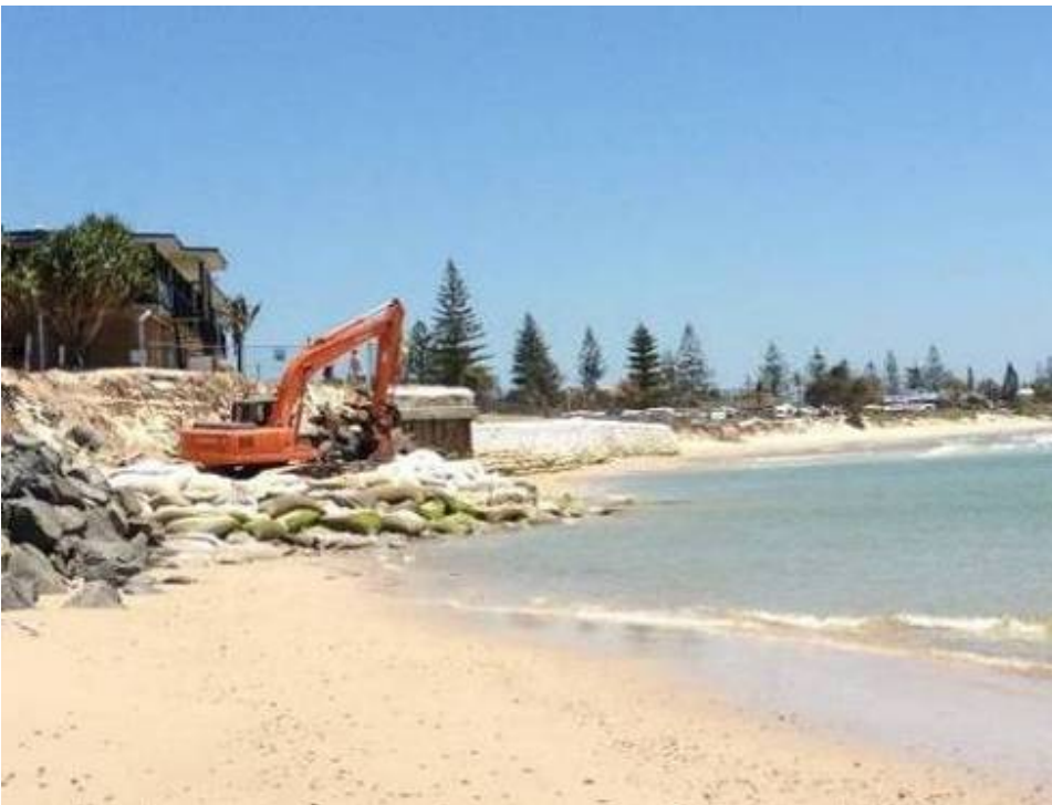
Figure 7 - Looking north from the terminal rock revetment towards Cudgen Headland SLSC and the Holiday Park showing both the piled concrete foundations and temporary geotextile sandbag wall. Photo: M Daley 8 November 2011.
