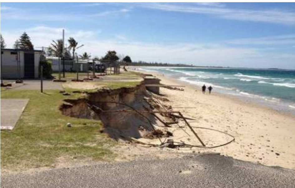
Figure 13 – Cable and Piping Infrastructure currents protruding from the erosion escarpment adjacent to the Holiday Park. Photo: M. Daley 8 November 2011.
