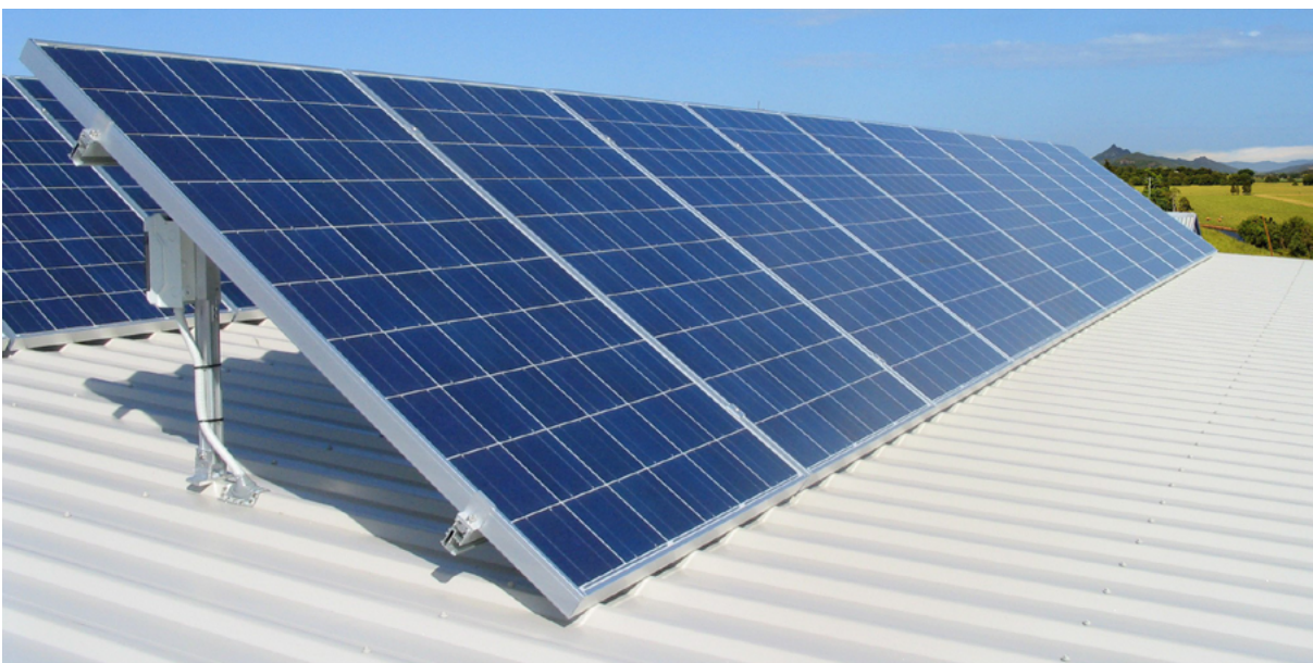
The Tweed has the highest uptake of rooftop solar in the Northern Rivers NSW
