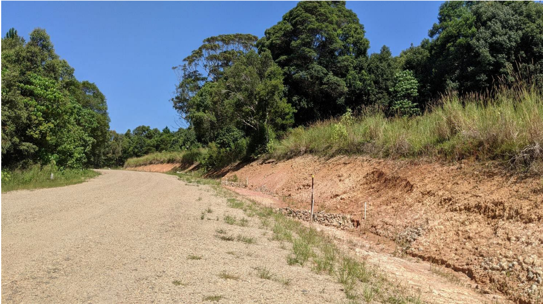
Figure 11: Rock check dams installed within table drains for erosion and sediment control.
