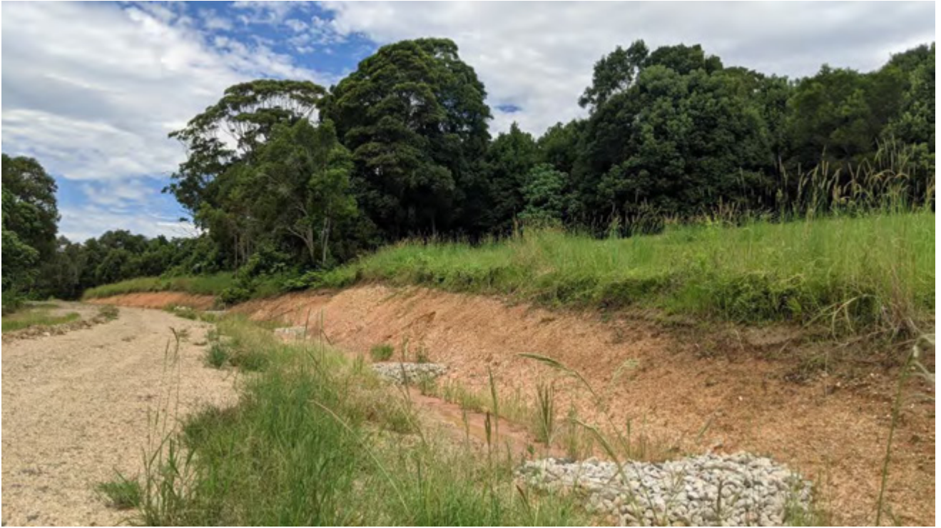
Figure 3: Rock check dams installed within table drains for erosion and sediment control.
