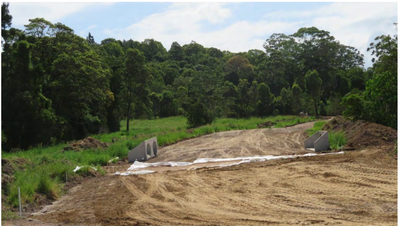
Figure 8 – Material placed within haul road alignment and drainage infrastructure in place ready for installation at approximately CH90.
