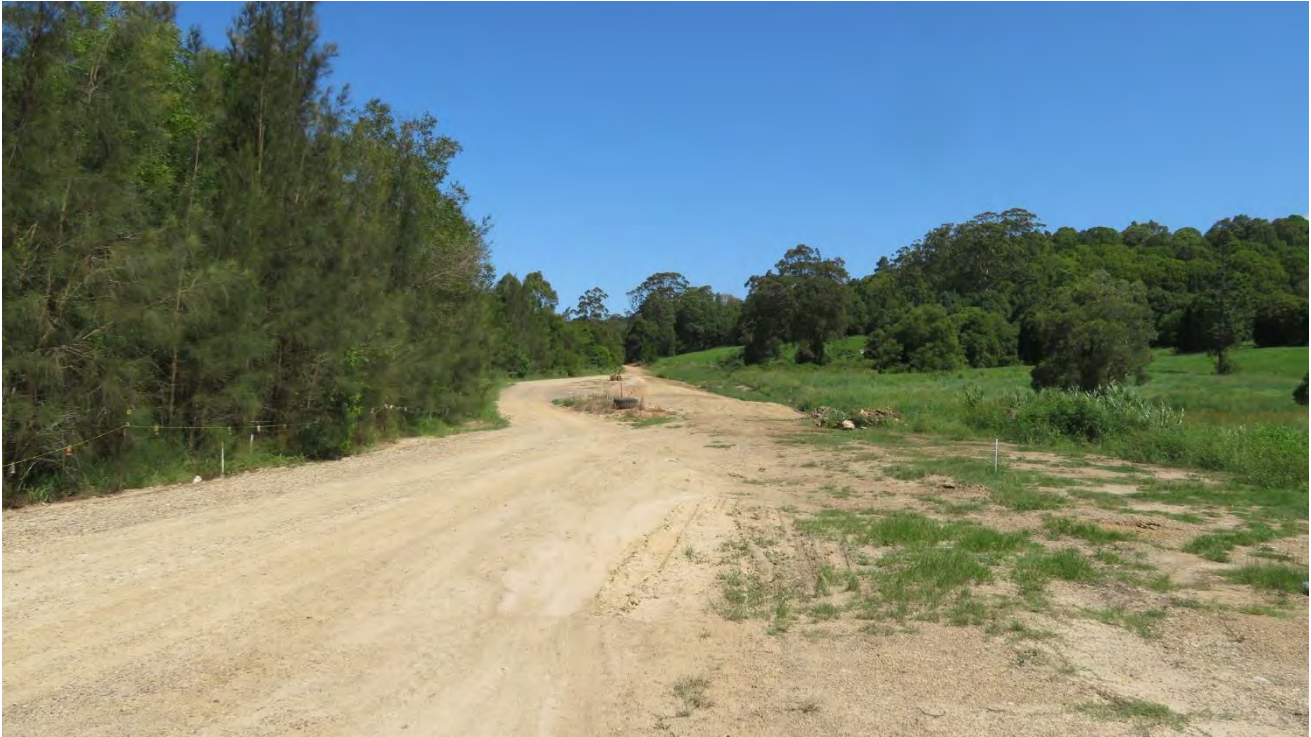
Figure 6 – Material placed within haul road alignment looking south between approximately CH700 and CH500.
