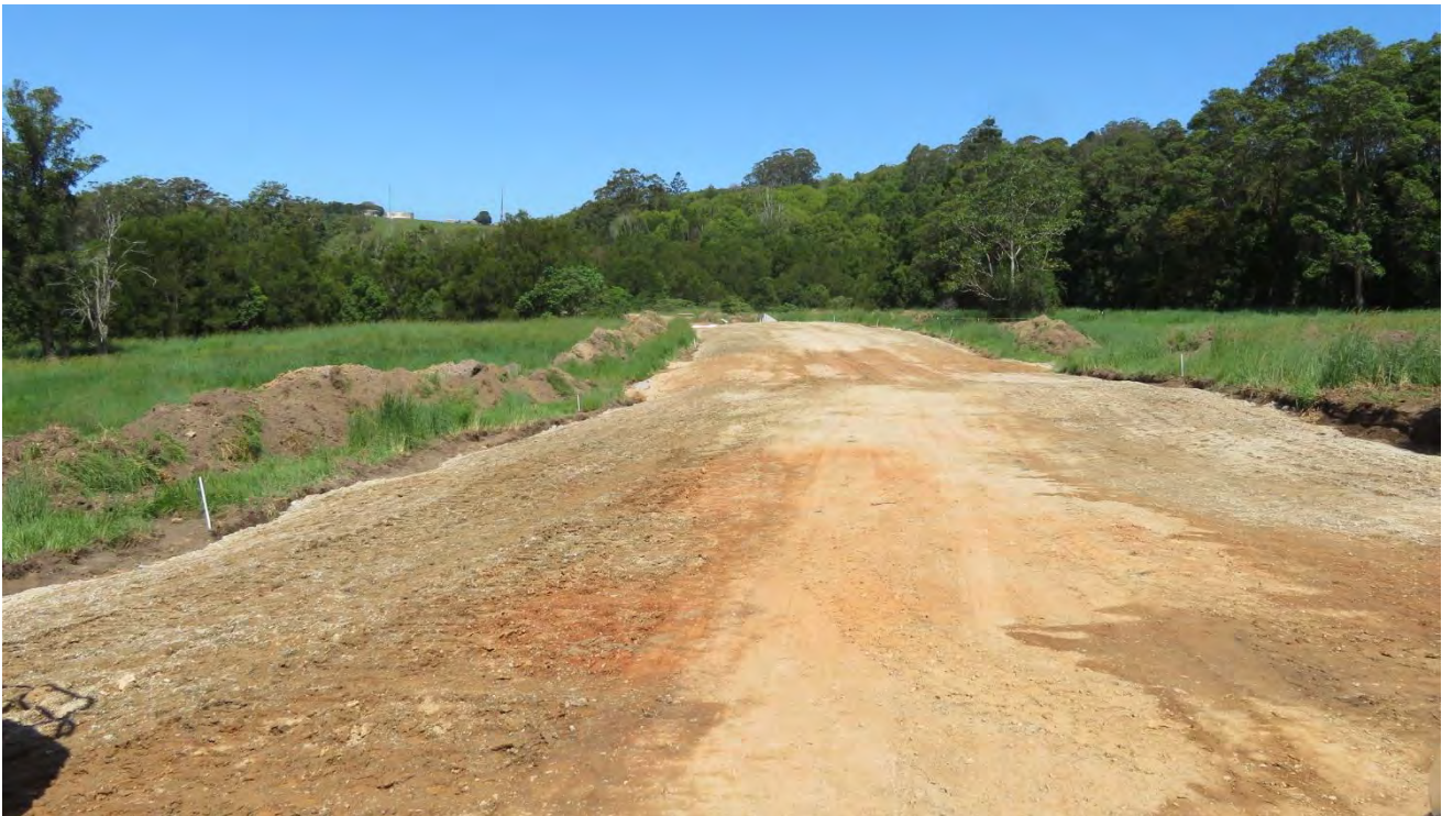
Figure 7 – Material placed within haul road alignment looking south between approximately CH300 and CH150.
