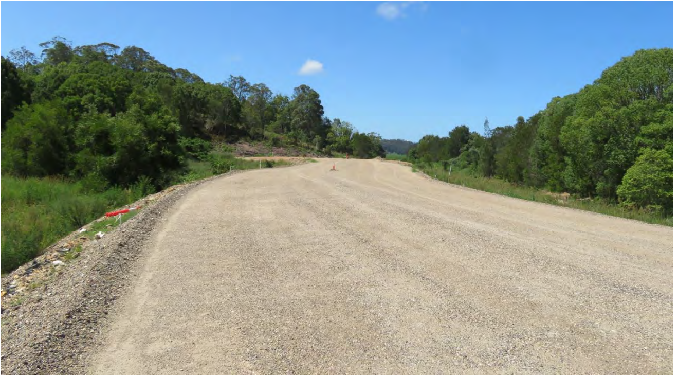
Figure 4 – Material placed within haul road alignment looking north between approximately CH800 and CH1000.
