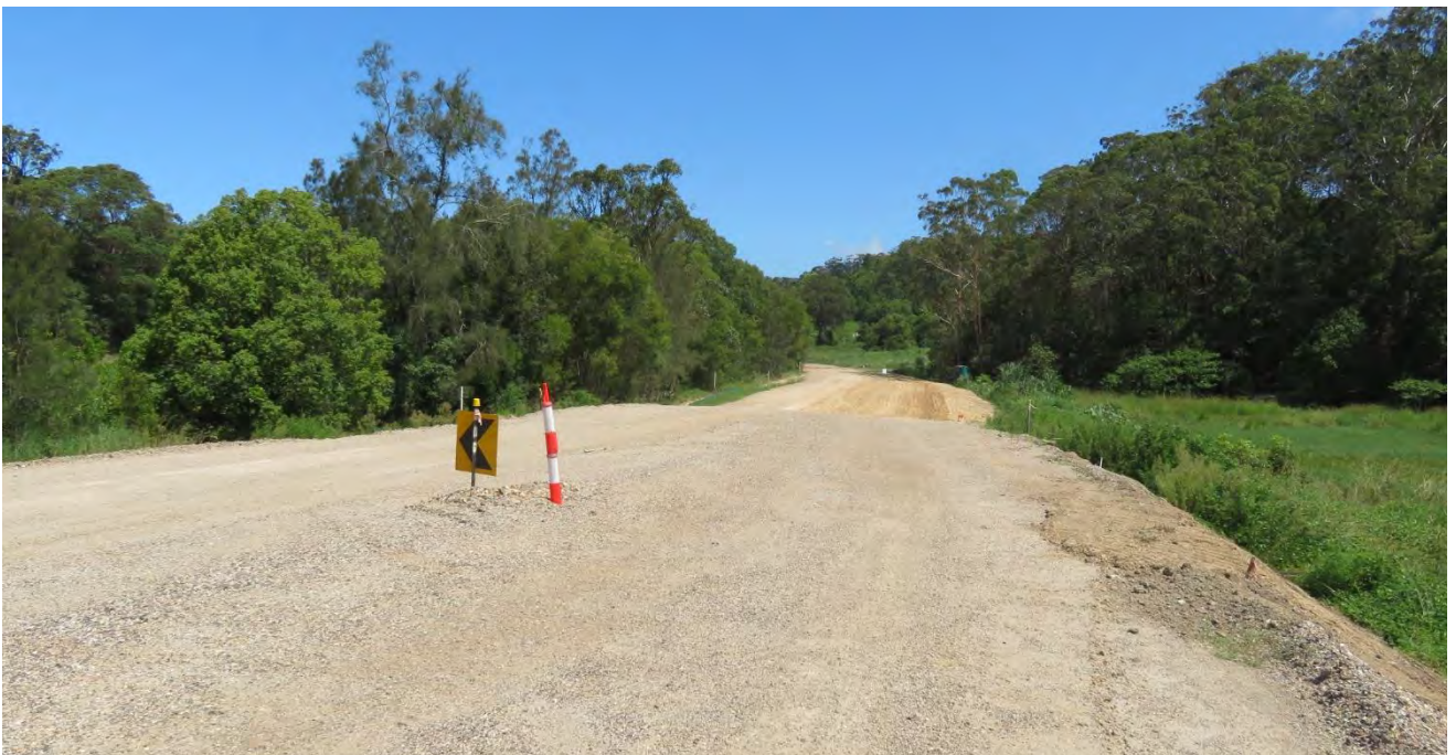
Figure 5 – Material placed within haul road alignment looking south between approximately CH800 and CH700.
