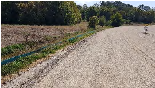
Photograph 3: Haul Road Settlement
