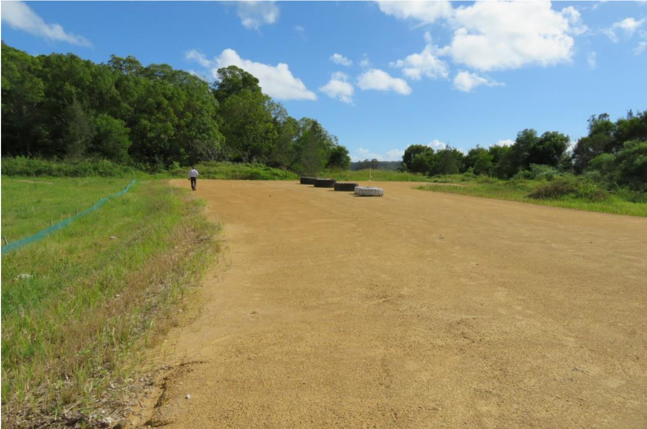
Figure 7 – Current haul road alignment following construction of the road base bridging layer between CH780 to CH1010 in preparation for future placement of fill above.
