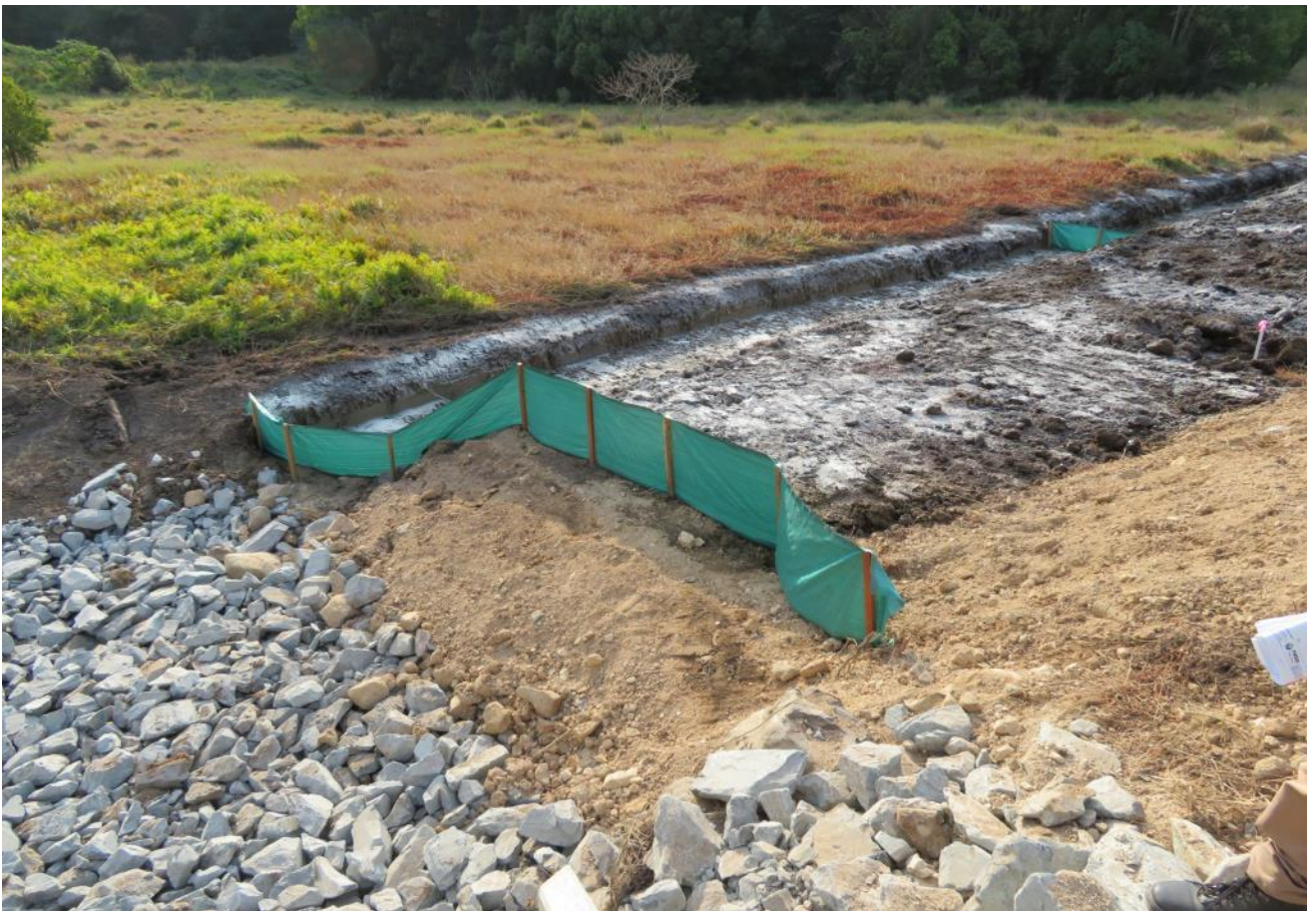
Figure 6 – Construction of temporary and permanent environmental controls associated with the construction of cross road culverts at approx. CH800.
