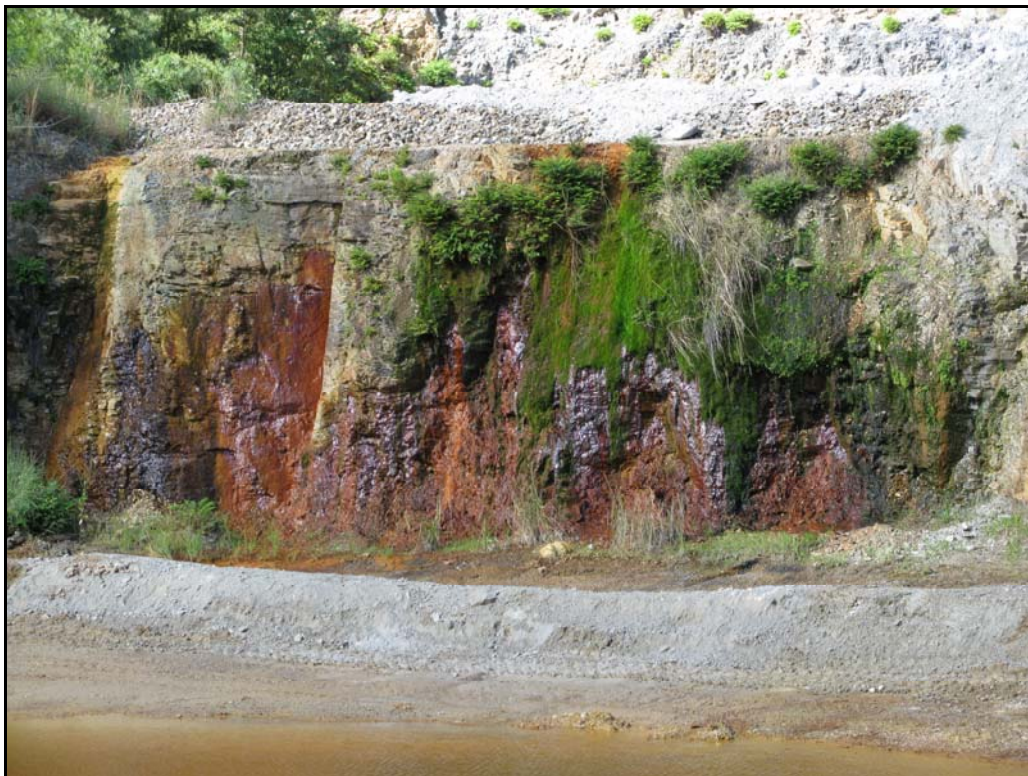
Figure 2: Seepage from exposed Bench 2 Batter above Sedimentation Pond
