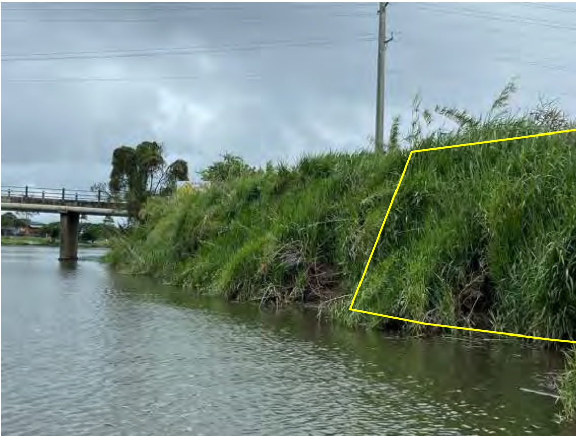
Plate 6: Disturbance footprint at the most southern end looking south along western bank to Cane Road bridge (yellow polygon indicates disturbance footprint)
