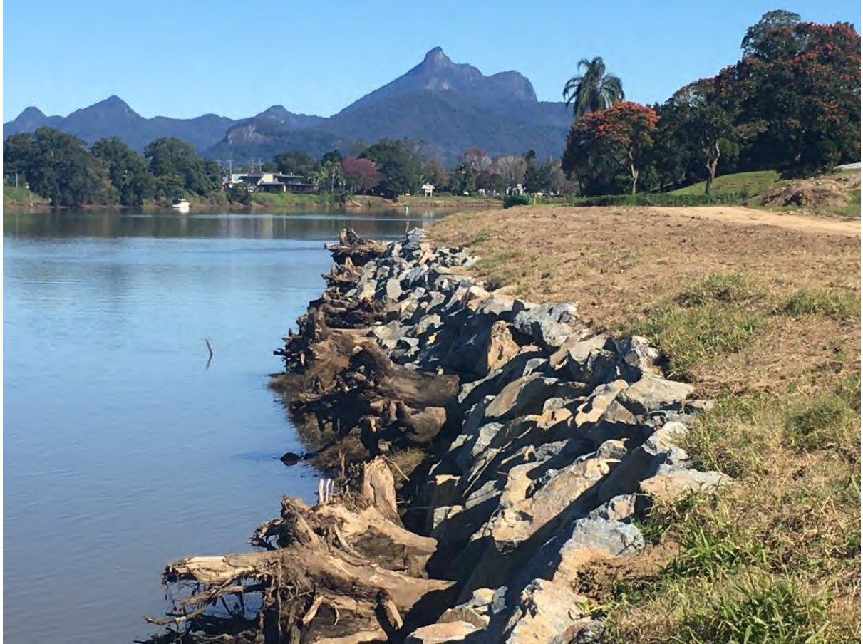
Example of completed fish habitat feature and rock revetment construction in Tweed River
