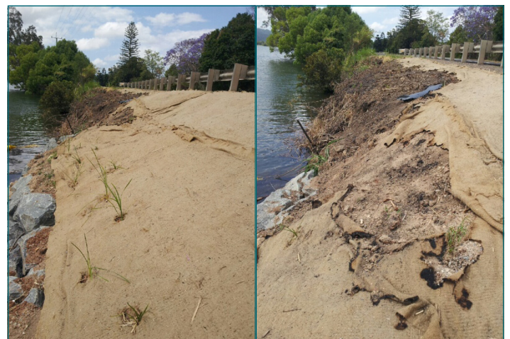
The partly-completed Lomandra planting adjacent to Tweed Valley Way, near Bartletts Road, Tumbulgum, before and after the vandal strike.
