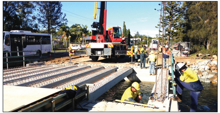
Workers continue to fit girders for the new Fingal Road bridge at Fingal Head. Next week they will begin to 'steel the deck' in preparation for the deck concrete pour the following week.
