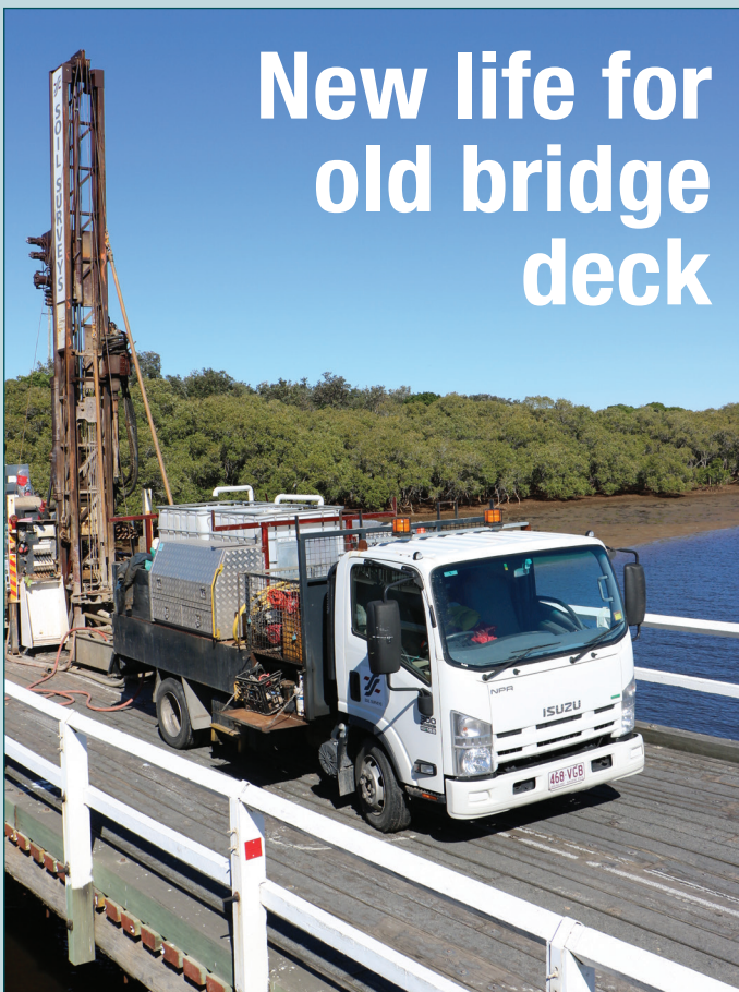
Contractors work from the old timber bridge deck to pre-drill the creek bed below at the central concrete pylon of the new bridge.
