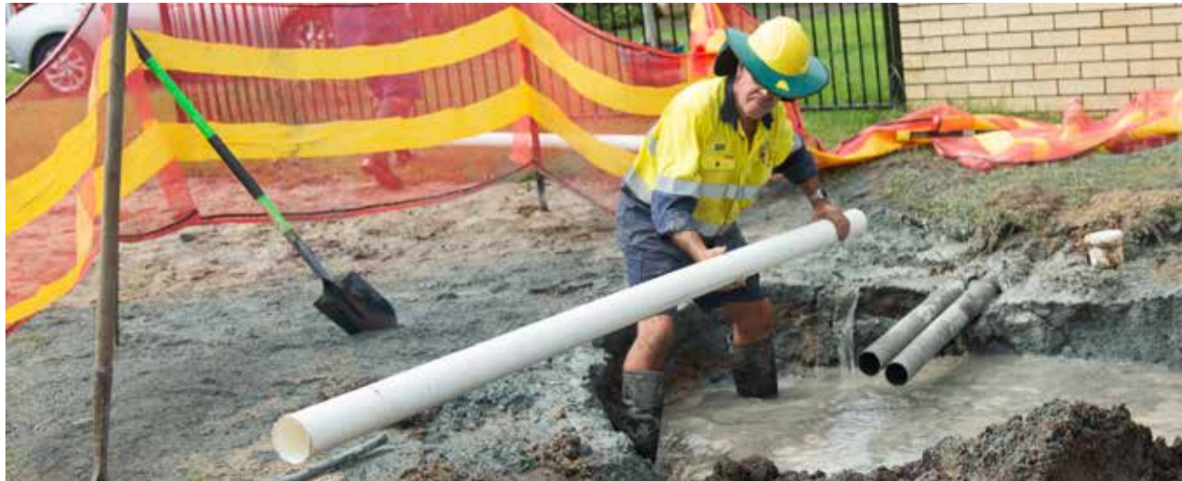
Tropical Cyclone Alfred temporarily knocked out a good portion of the Tweed's water supply, but Council's Water and Wastewater crews weathered the blows to get infrastructure back on its feet.
