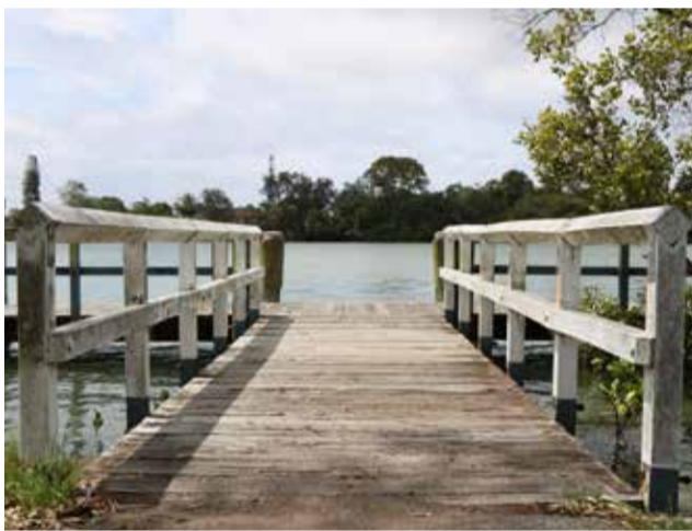
Works to enhance facilities at Dry Dock Road boat ramp will be commencing soon.
