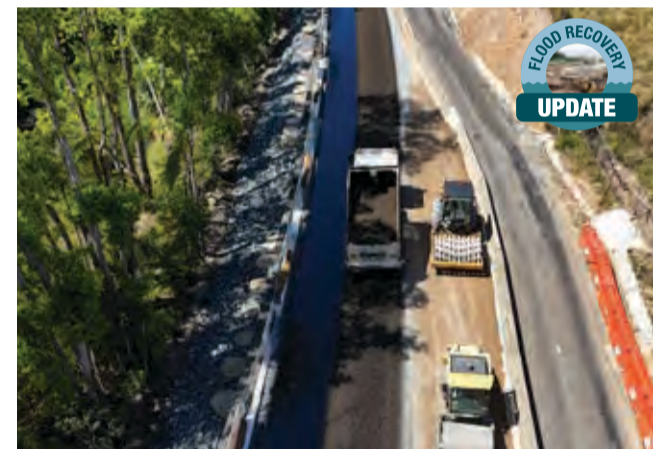
Road sealing underway on the eastbound lane at the slip site on Tyalgum Road.
