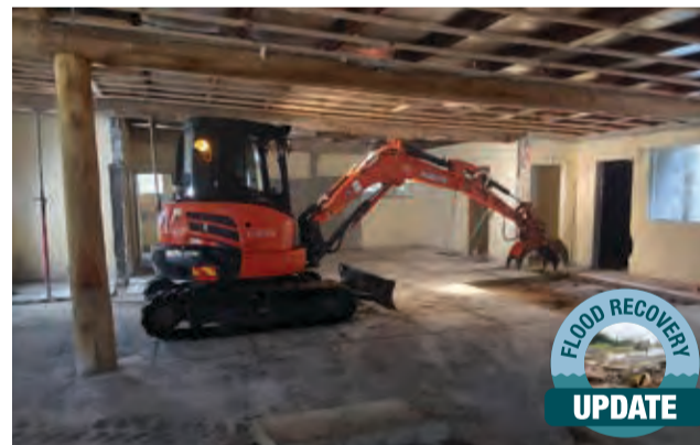
Demolition works are underway at the Vic Bianchetti Sports Grounds at Uki.
