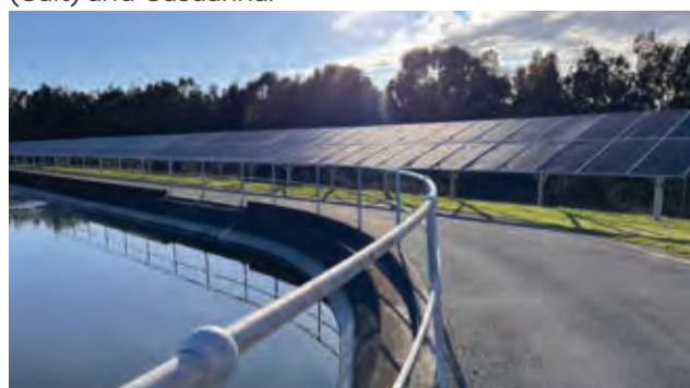
Council has installed an extra 160 solar panels at the Kingscliff Wastewater Treatment Plant.
