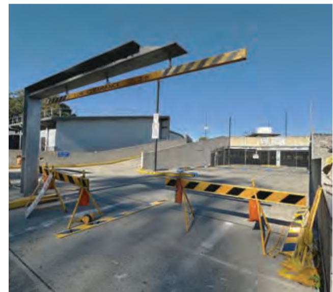
Entry to the top levels of the Murwillumbah multi-level carpark has been closed since December following a vehicle fire.
