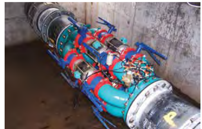
Council's pressure reduction valves help achieve more consistent water pressure across our water supply networks.
