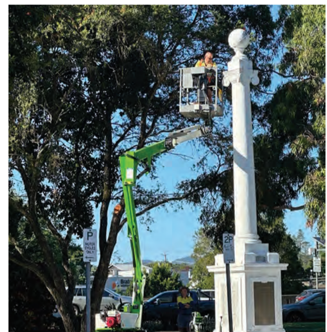
Council staff repainting the ANZAC Memorial at Remembrance Place, Murwillumbah ahead of ANZAC Day.
