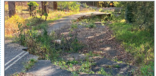
Part of the extreme landslide on Tyalgum Road.
