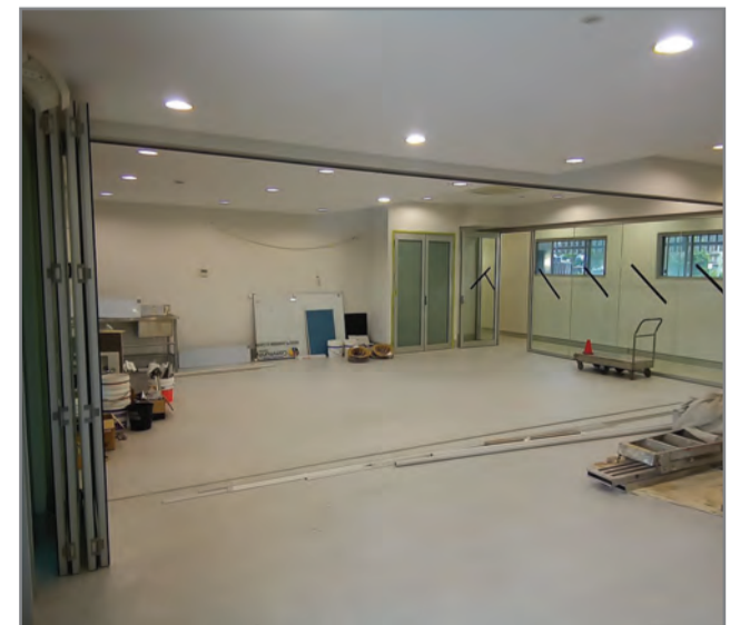
Bi-fold doors have been installed in a main meeting area at the Murwillumbah Community Centre, with epoxy flooring and wall painting completed.
