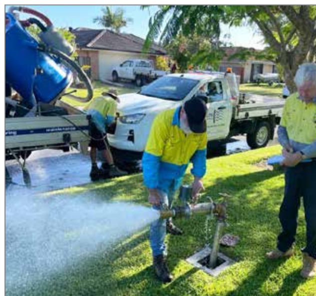
By mid-March, Council's contractor Clearflow will have cleaned the water mains at 8 Tweed locations.
