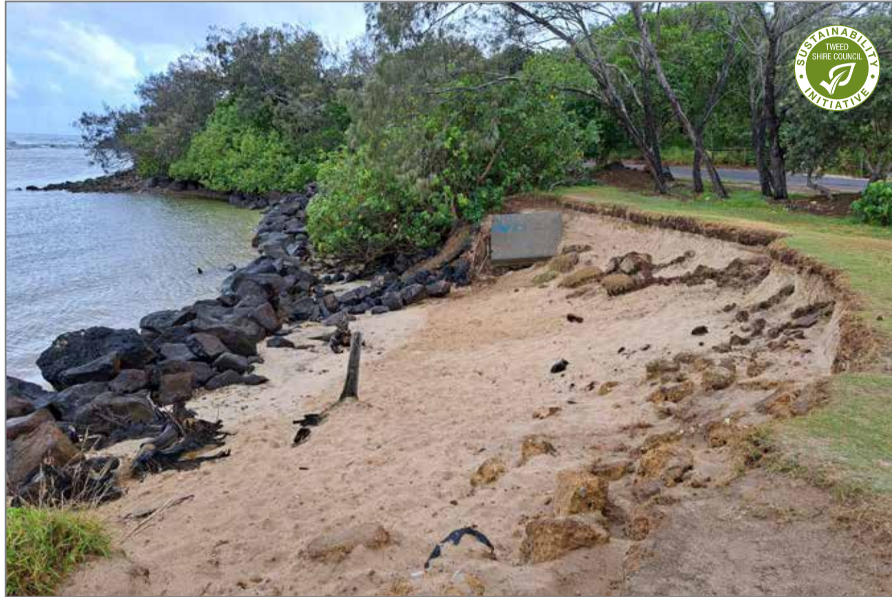
Repair works will commence at Cudgen Creek, Kingscliff to prevent further erosion at the site as pictured.
