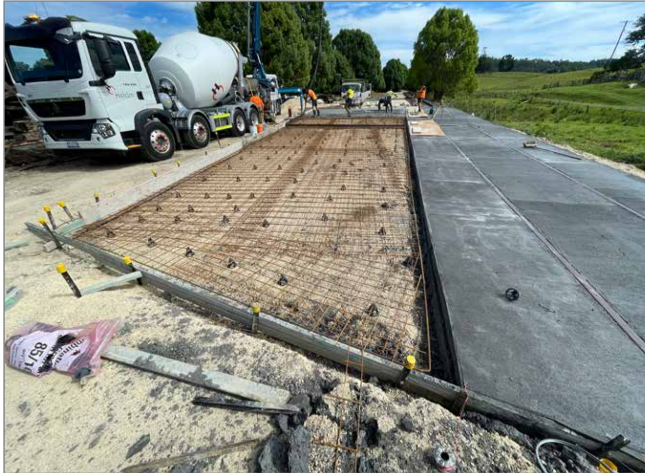
Workers constructing the slab to mark the old station at Dunbible. Work is continuing along the Tweed leg of the Northern Rivers Rail Trail, which is expected to be open to the public early next year.
