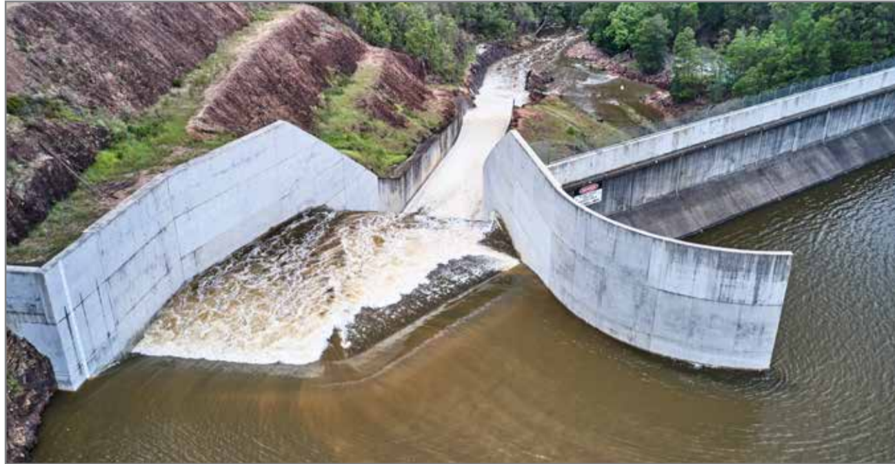
As the Clarrie Hall Dam fills during intense rainfall events, it is designed to safely pass the excess water into Doon Doon Creek and then the Tweed River. This spilling cannot be controlled.
