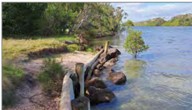
One of the degraded sections of retaining wall along Mooball Creek at Pottsville to be repaired.
