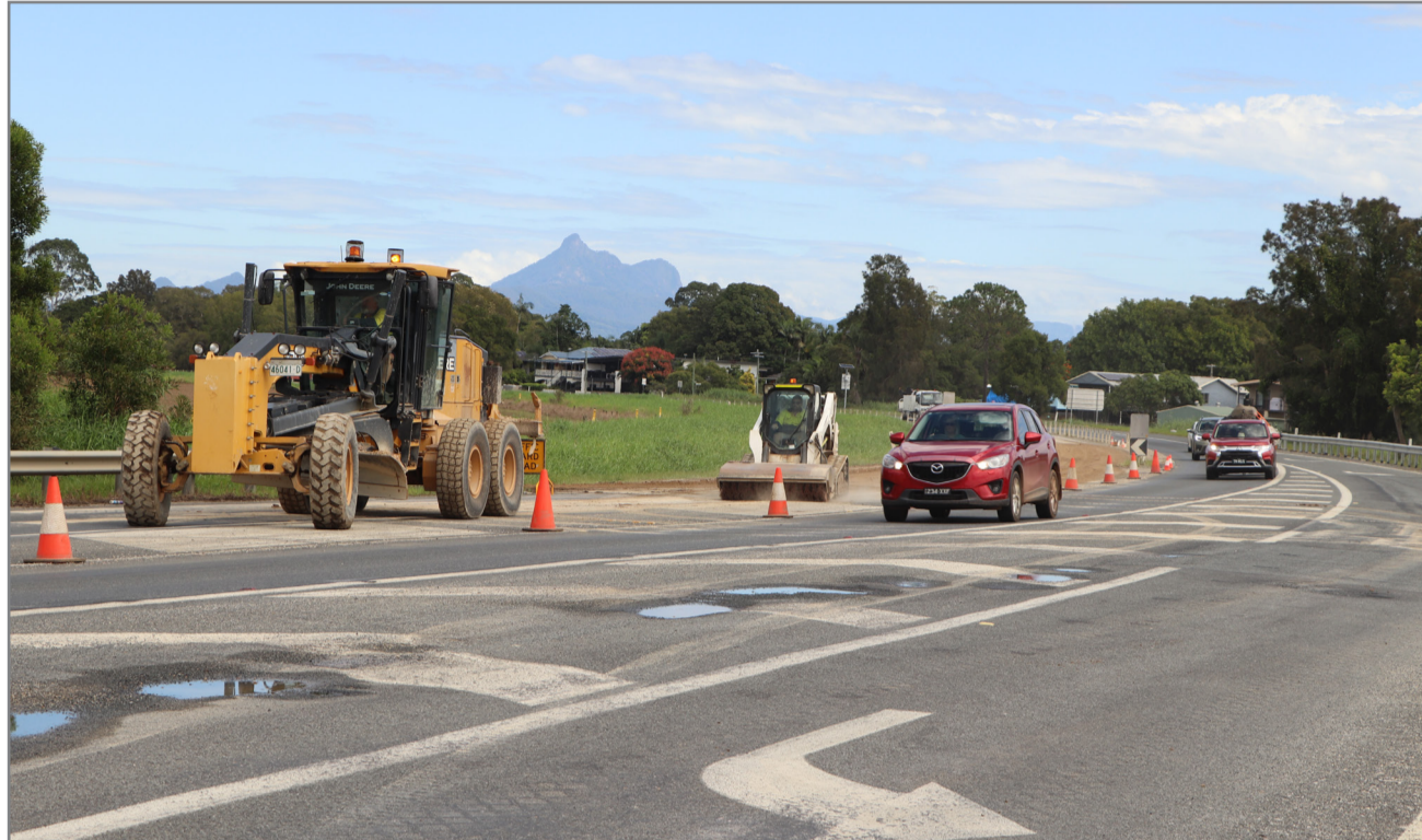
Permanent roadworks have begun on Tweed Valley Way, near the Tumbulgum Road intersection, which suffered significant damage in the floods. Nightworks are taking place in this area to minimise disruption.
