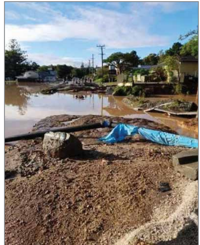
Tweed Valley Way has collapsed at Blacks Drain at South Murwillumbah, damaging water and sewer connections and leaving nearby residents without water.
