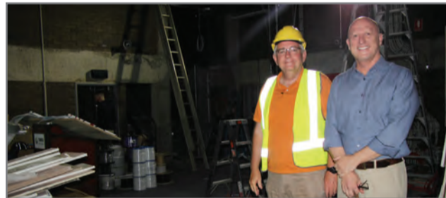
Colin Elliott (left) inspects the 'work in progress' with Council's Andrew Illingworth, Manager Tweed Holiday Parks and Cultural Facilities.
