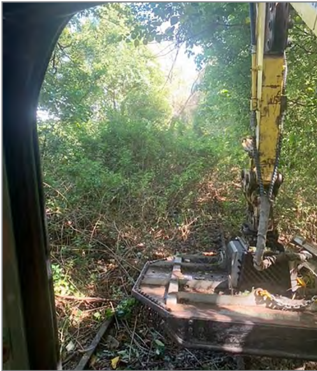
Clearing the way to design and construct the Tweed section of the Northern Rivers Rail Trail.
